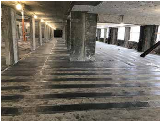
Fig. 7: The hallway and room slabs after the CFRP installation, focusing on the 8 in (200 mm) wide application
