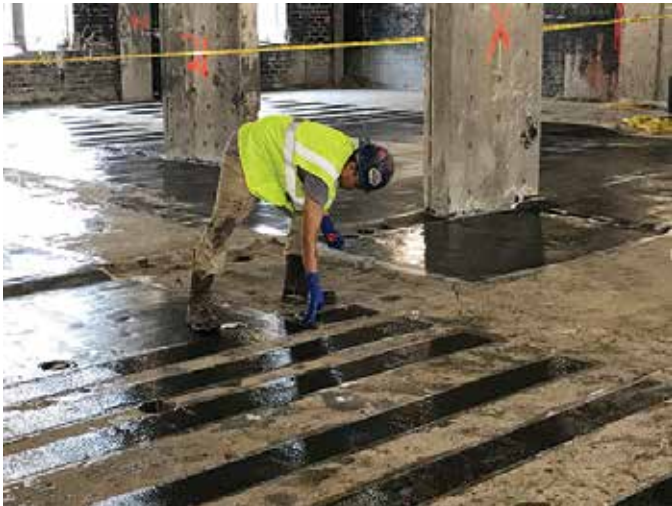
Fig. 6: Installing the final epoxy resin layer for CFRP (also performed to “knock down” any fiber edges)
