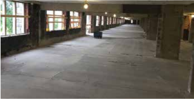
Fig. 2: Barrack slabs prepared by shotblasting before installing the crack infills and CFRP
