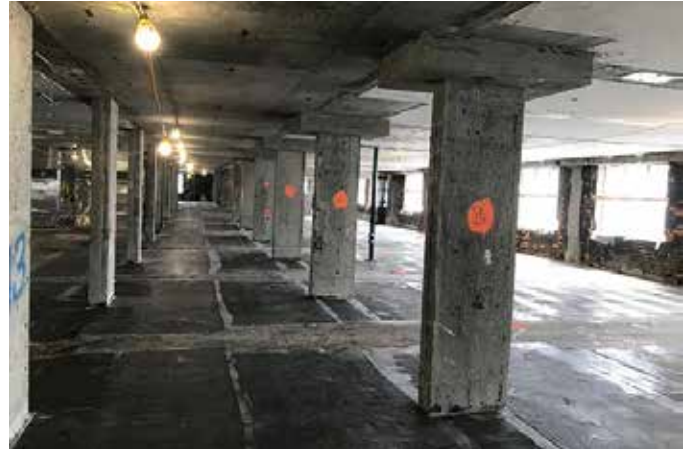
Fig. 8: The hallway and room slabs after the CFRP installation, focusing on the 50 in (1270 mm) wide application
