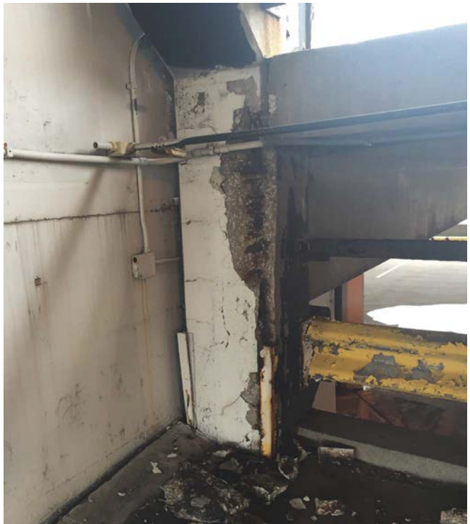
Fig. 2: Existing condition discovered at an interior column
