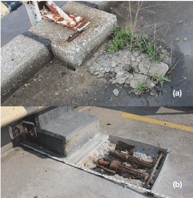
Fig. 5: (a) Many grout pockets on the roof were delaminated and some had vegetation growing, and (b) Grout pocket after concrete removal and cleaning
