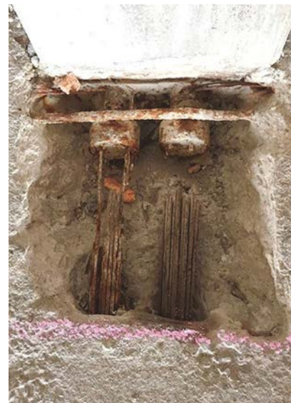
Fig. 3: Many beams were observed to have completely corroded through tendons
