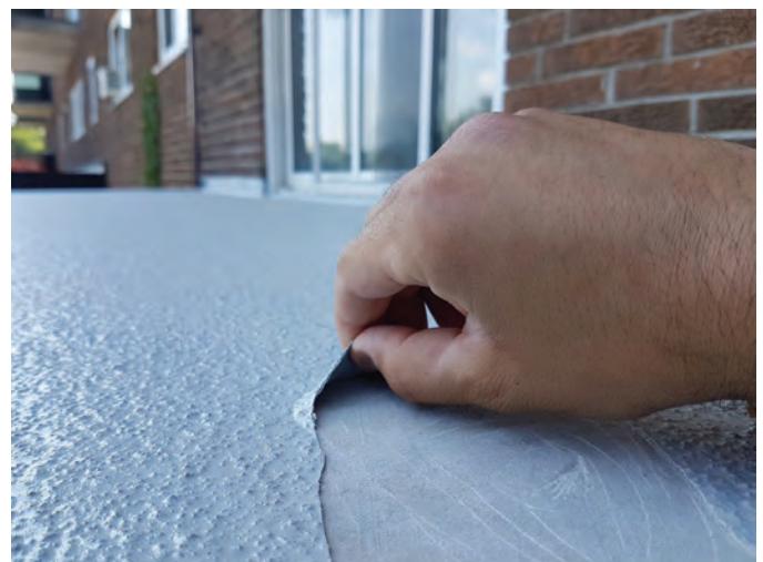
Fig. 2: Debonded waterproof membrane due to excessive moisture in balcony slab
