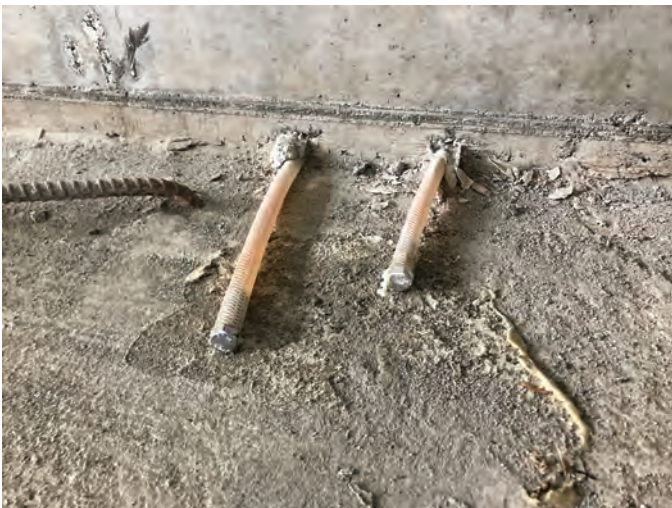
Fig. 10: Injection grouting, typically specified in Division 03, can play an important role in a building’s waterproofing solution as both a corrective measure and as an injectable waterstop (photo courtesy of DTR Consulting Services)
