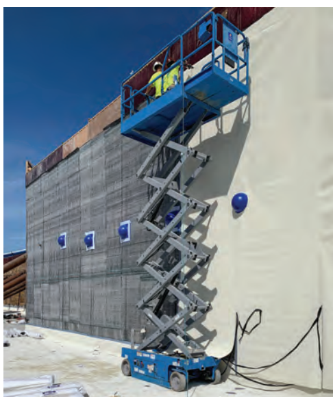
Fig. 4: Condition 15a Shored Blind-side Wall – Hydrostatic (Shotcrete); a dual waterproofing system was used, combining Section 07 13 26 - Self-Adhering Sheet Waterproofing with Section 07 17 16 - Bentonite Composite Sheet Waterproofing (photo courtesy of AVM Industries, Inc)
