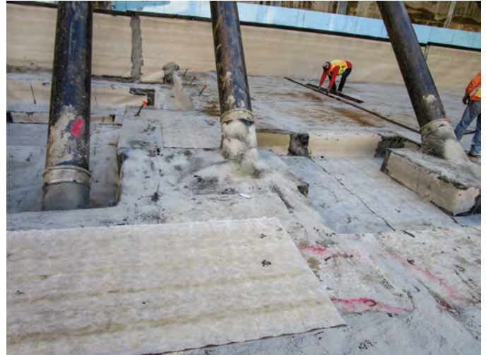
Fig. 8: Rakers, the braces used to temporarily support foundation walls, will be removed after the grade-level floor plate is constructed, leaving gaps in the waterproofing that will have to be repaired (photo courtesy of Simpson Gumpertz & Heger)
