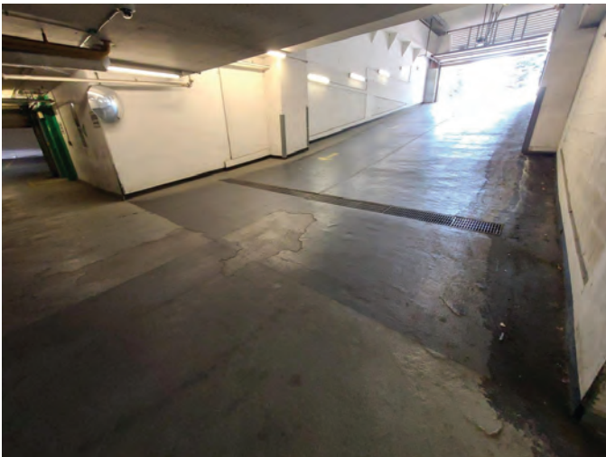
Fig. 5: Lateral movement of moisture in slab from trench drain causing debonding of the surrounding membrane coating
