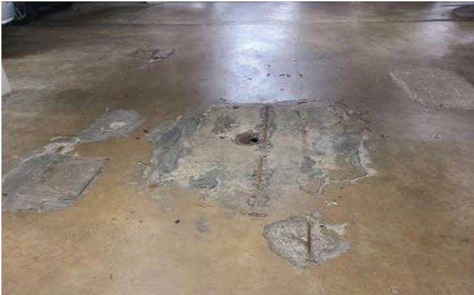
Fig. 3: Top surface delamination with exposed reinforcing steel in an elevated garage deck slab during a condition assessment
