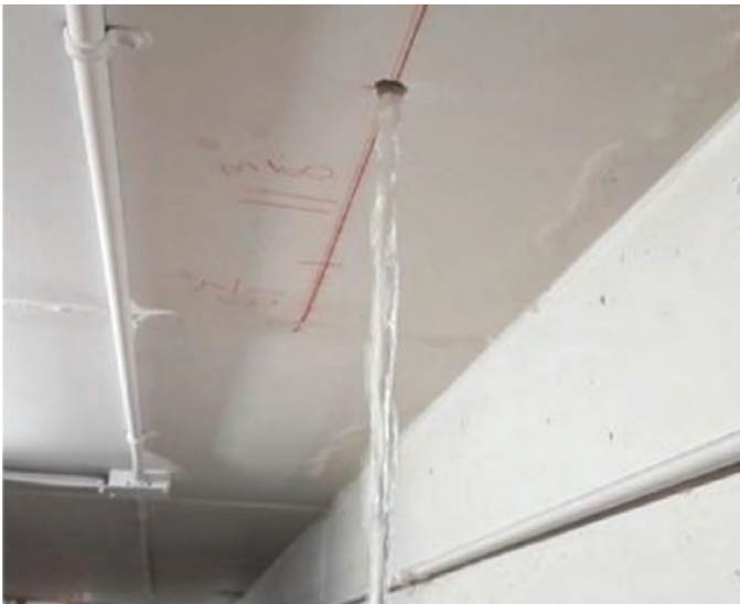
Fig. 4: Trapped water pouring from vent hole installed at the soffit of a hollow core slab
