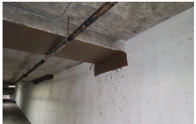
Fig. 8: Crystalline coating applied below a garage ramp trench drain and wall upturn
