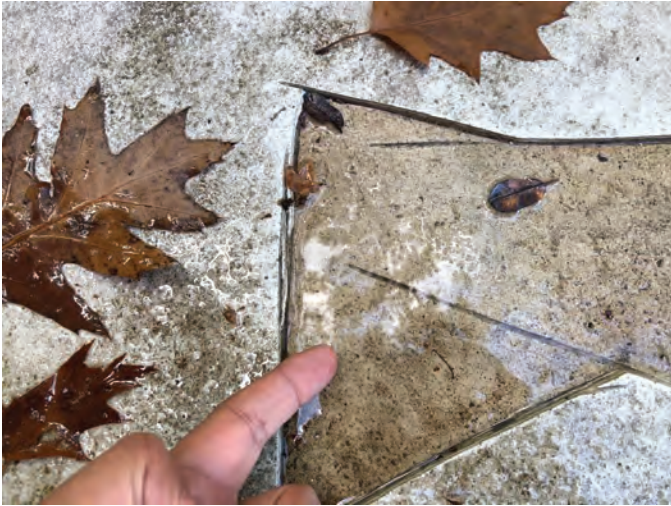
Fig. 3: Trapped moisture below waterproof membrane due to unvented composite steel deck
