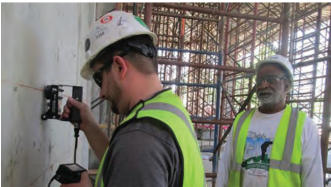
Fig. 5: Conducting impact-echo tests on a reinforced concrete shear wall to detect honeycombing and voids
