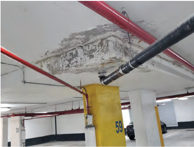
Fig. 9: Water penetration at an expansion joint and drain in a newer building
