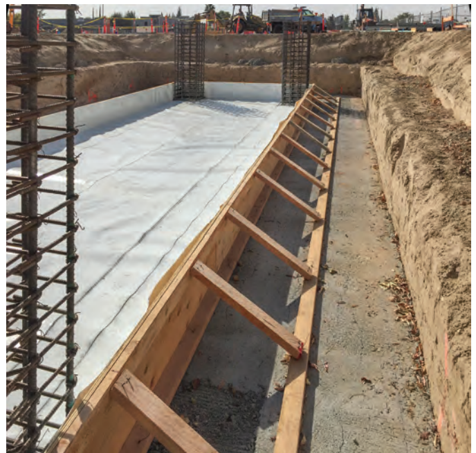
Fig. 9: Thermoplastic sheet waterproofing installed before reinforcing steel—manufacturers typically require inspections after the initial membrane installation and after reinforcing steel has been placed to check for trade damage (photo courtesy of DTR Consulting Services)
