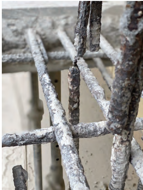
Fig. 3: The rebar in many of the repair areas were found to be unbonded and corroded beyond repair
