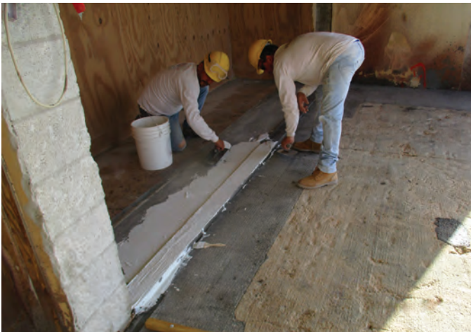
Fig. 5: All window and door openings were redone, and additional waterproofing was added to ensure future protection from leaks
