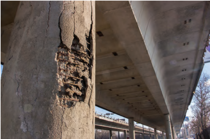
Corrosion of steel reinforcement embedded within concrete due to the ingress of chlorides from deicing salts or salt air is a major cause of bridge deterioration
