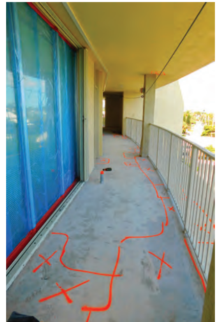
Fig. 4: Repair areas marked after NDT such as hammer tapping and chain dragging were performed to determine extent of required repairs
