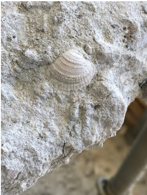
Fig. 2: A close-up of one of the seashells found within the concrete matrix of the building structure
