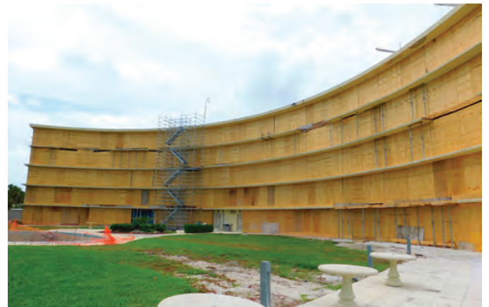
Fig. 8: Hamilton House had to be completely boarded up as Hurricane Dorian threatened the Florida East Coast during the height of repair work, creating many logistical challenges
