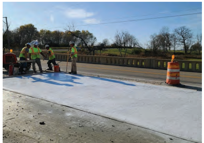
Bridge deck overlays using UHPC can protect underlying structural concrete from chloride ingress (photo courtesy of Steelike)
