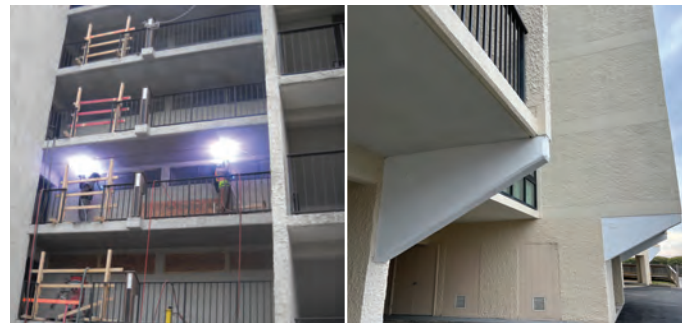
Fig. 10: Thermal spray being applied to the PHCP soffits (left) and current condition of haunches after thermal spray and coating application (right)
