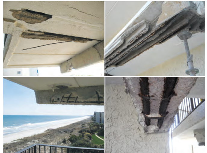
Fig. 2: Corrosion damage: prestressed hollow core panels at Level 1 walkway soffit (top left), balcony prestressed hollow core panel during construction demolition (top right), balcony cantilever beam (bottom left), and walkway beam (bottom right)
