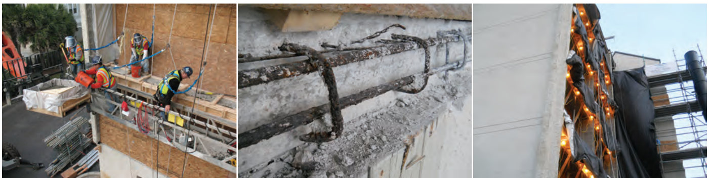
Fig. 5: Replacement of balcony slab edges from swing stage (left), example of corrosion of reinforcing steel during demolition (center), and example of thermal control (right)
