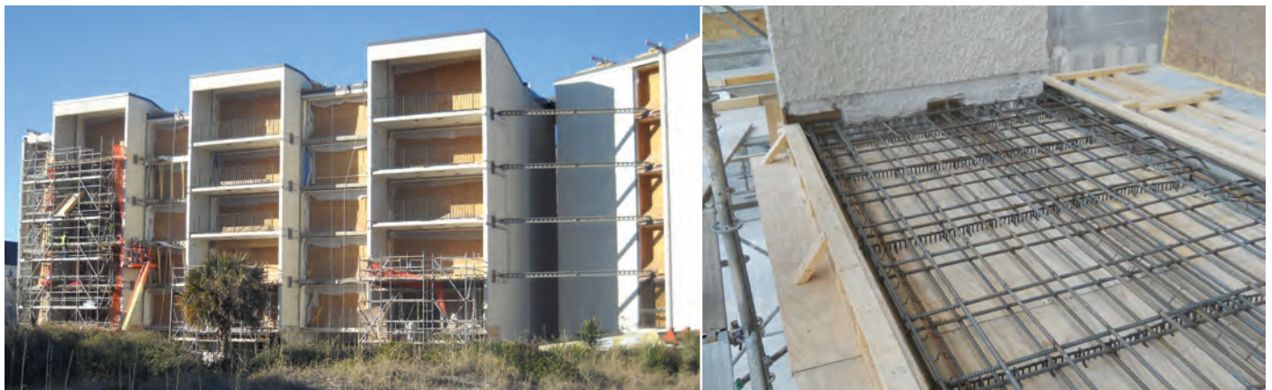
Fig. 6: Lateral bracing necessary for removing balcony slabs (left) and reinforcing layout at balcony (right). Note tabs at privacy wall used to support the new slab. Not easily visible in the figure is the tab nearest the threshold
