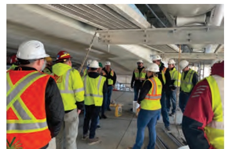
Attendees are seen here with Blake Rago, from RH Ward & Associates, as he talked about the extensive restorations while on the suspended scaffold
