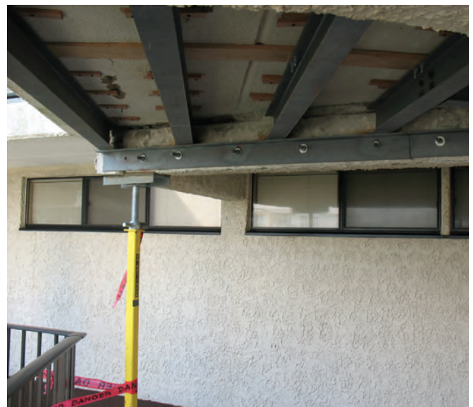
Fig. 3: Example of supplemental supports prior to project to make conditions temporarily safe
