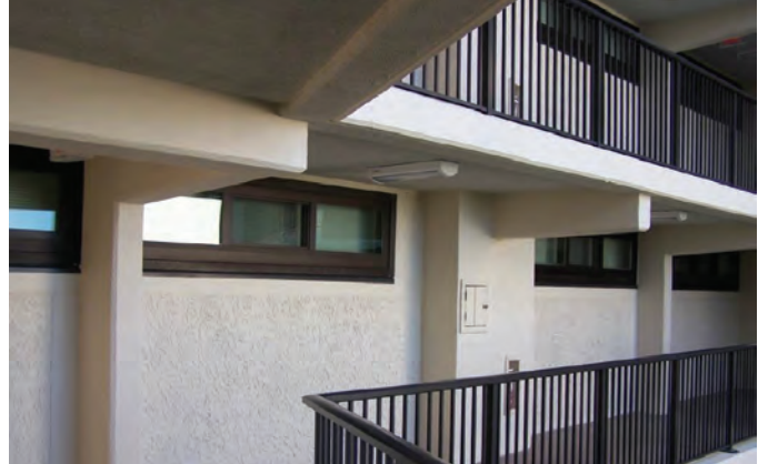
Fig. 9: Walkway cantilever beam showing removed concrete, low cover to bottom of beam, excessive cover to top tension reinforcing steel, and voids (top left), partially placed and formed reinforcing steel for reconstructed beams and pilasters used to reduce the stresses in the beam (top right), and completed pilasters and beams cast integrally with the new concrete slabs (bottom). The pilaster was tied to the wall. Note the mechanical splices used to tie to existing steel for this beam.
