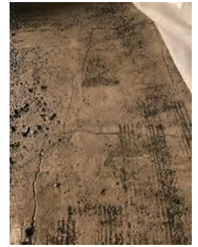
Fig. 6: Insufficient substrate preparation (photo courtesy of Jensen Hughes Inc.)
