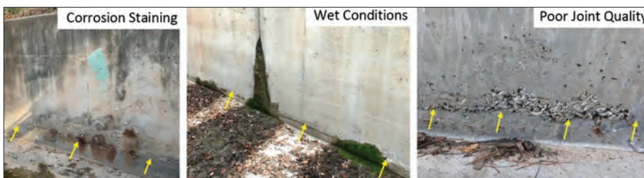
Fig. 5: Visual observations indicating an elevated risk of localized corrosion at the joint (yellow arrows).
