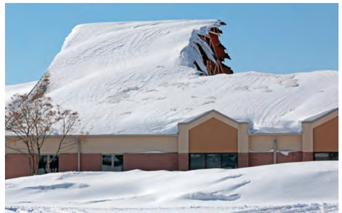
Fig. 3: Structural failure due to the heavy snow (Photo: www.twincities.com)
