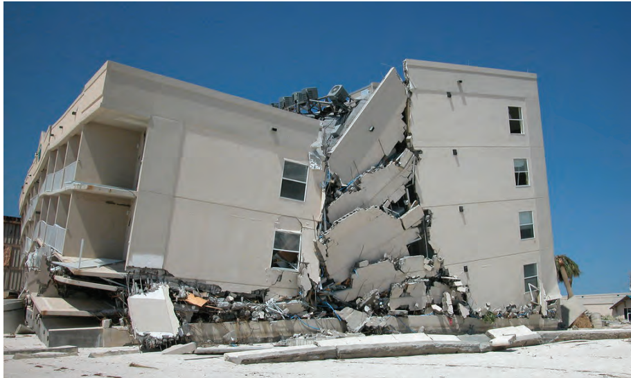
Fig. 1: Structural failure of a concrete structure (Photo: TEEX, www.flickr.com/photos/teex/4166709041 )
