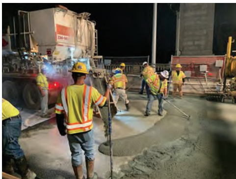
Fig. 1: Installation of a bonded cementitious overlay (photo courtesy of Jensen Hughes Inc.)
