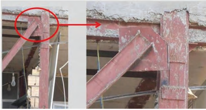
Fig. 4: Insufficient welding on the gusset plate observed on site
