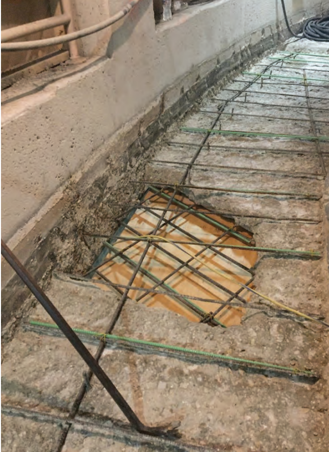
Fig. 4: Localized full-depth concrete repair within the limits of the bonded overlay (photo courtesy of SK&A)
