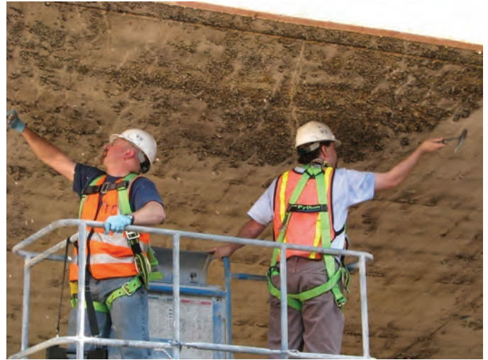
Fig. 4: Sounding is sometimes useful in identifying concrete damage, e.g. incipient spalling or weakened concrete. Photo source: Wiss, Janney, Elstner Associates, Inc.
