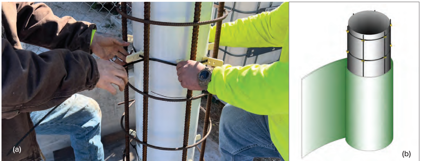
Fig 2: Spacers being installed (a) and the FLF laminate being wrapped around a deteriorated column (b)
