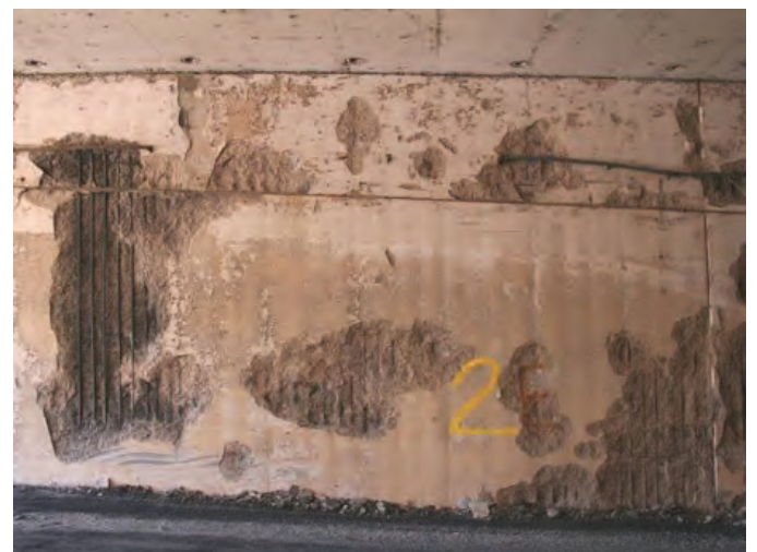
Fig. 10: Concrete spalling was extensive in areas with severe exposure to the fire. Photo source: Wiss, Janney, Elstner Associates, Inc.
