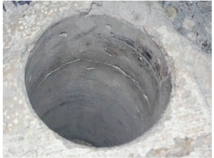
Fig. 11: Large scale, blind deep delaminations were found in some panels tested. Photo source: Hydropressure Cleaning, Inc.
