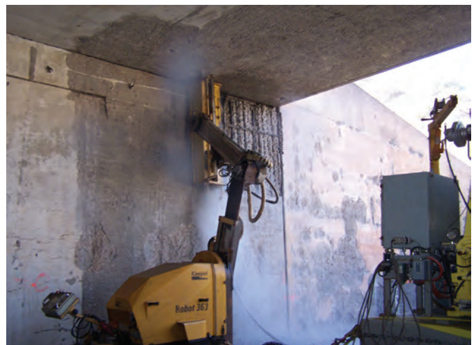
Fig. 13: The unique Multipurpose Arm (MPA) allows hydrodemolition contractors to easily attack horizontal, vertical, overhead and below-track surfaces, all at the push of a button. Photo source: Hydropressure Cleaning, Inc.
