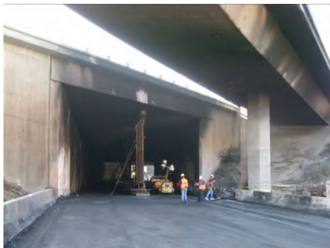
Fig. 8: Soot blackening was present on the South exit of the Tunnel where the accident occurred. Photo source: Wiss, Janney, Elstner Associates, Inc.
