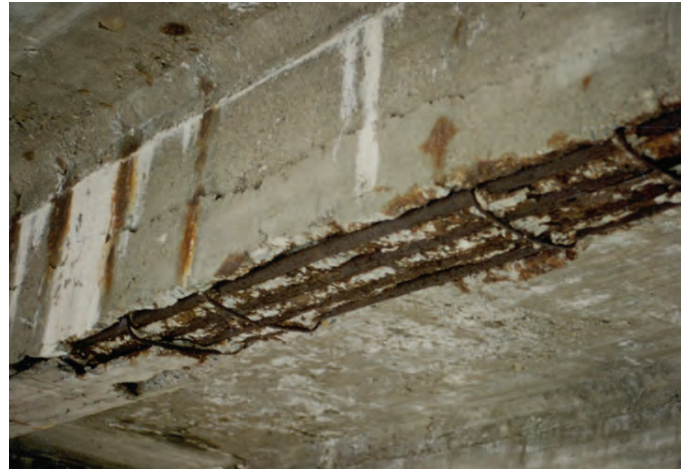
Fig. 8: Deterioration of reinforced concrete half joint (courtesy of SIMCO Technologies)
