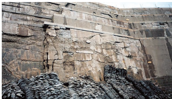
Fig. 3: Deteriorated concrete near expansion joint
