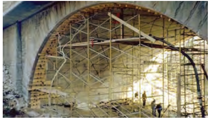
Fig. 6: Form and Pour application on concrete arch bridge (courtesy of D.W. Fowler)
