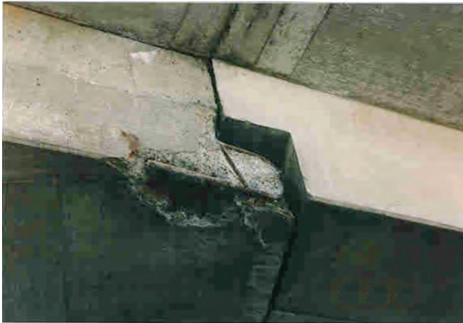
Fig. 7: Deterioration of a reinforced concrete beam due to corrosion (courtesy of Transports Quebec)
