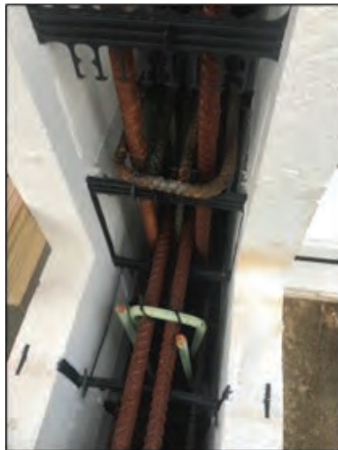
Fig. 8: Multiple rebar closely stacked together
