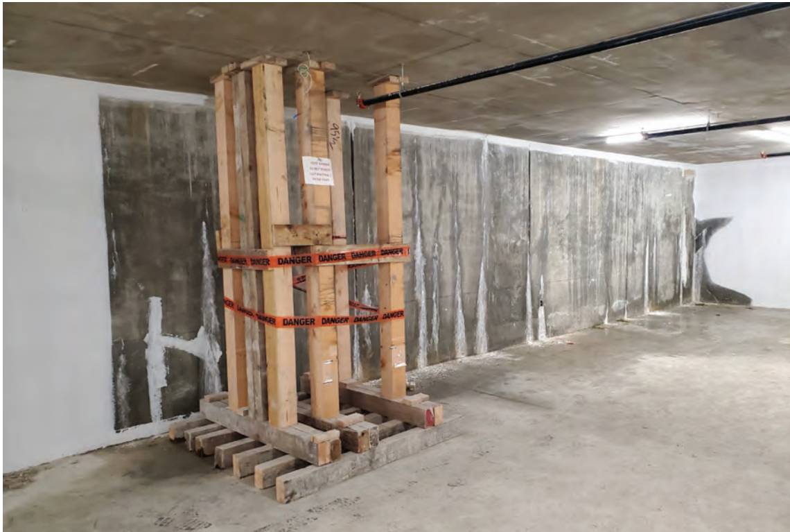
Fig. 1: Cast-in-place concrete structural walls in need of leak repair
