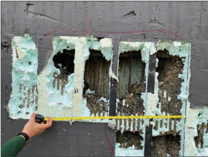
Fig. 5: Void exposed after removing insulation at suspect location identified using GPR scanning
