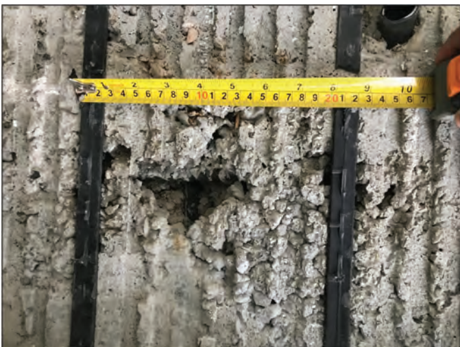
Fig. 7: Small void exposed using GPR scanning
