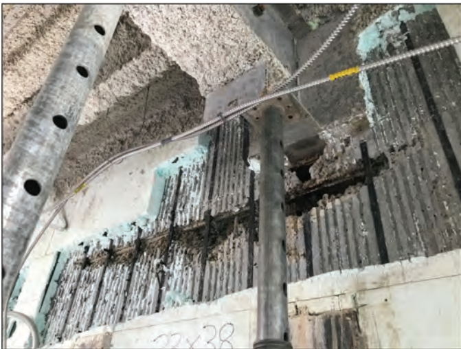
Fig. 6: Void exposed using GPR scanning
