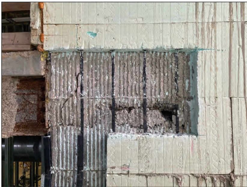
Fig. 2: Void and cracking at a typical ICF wall
