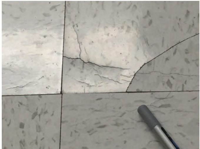
Fig. 3: Cracked and warped flooring (photo courtesy of Concrete Science, Inc.)
