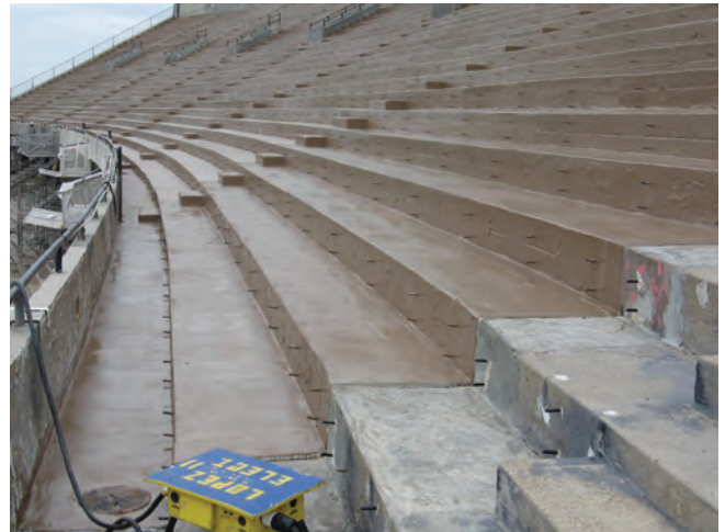
Fig. 3b: Concrete surfaces at the Upper Deck protected by pedestrian traffic deck coating system
