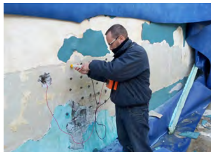
Fig. 5: Condition assessment included a corrosion potential
