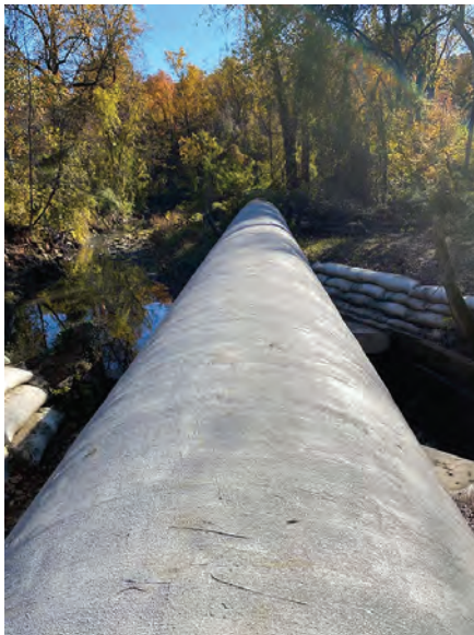
Fig. 7a: A view of the aerial sewer from above, spanning across the Hickey Run Creek
