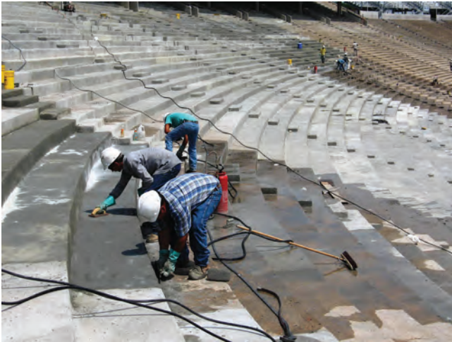
Fig. 3a: Applying cementitious overlay to horizontal and vertical surfaces at the “Lower Bowl”
