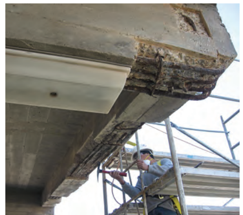
Fig. 2: Sounding of concrete at underside of Upper Deck prior to installation of repair mortar
