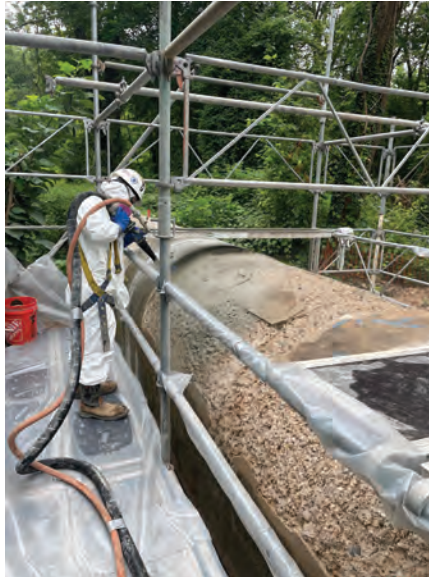
Fig. 5: To prevent dust generation and potential contamination of the stream, crews used garnet mist blasting instead of sandblasting
