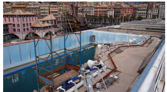
Fig. 3: The waterproof coating was unable to prevent chlorides from penetrating deep into the concrete
