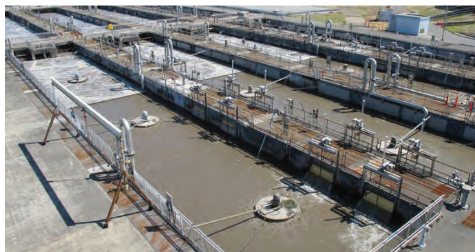
Fig. 1: Aerial view of the aeration basins during operation
