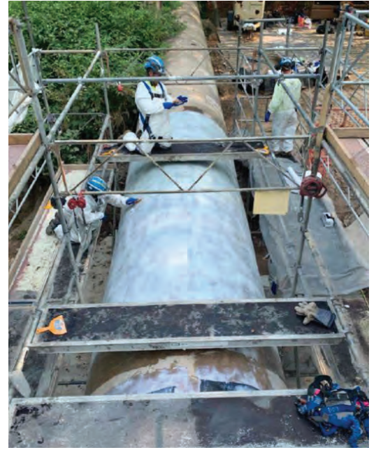
Fig. 3b: Crews installed CFRP and GFRP systems on the exterior of the aerial sewer
