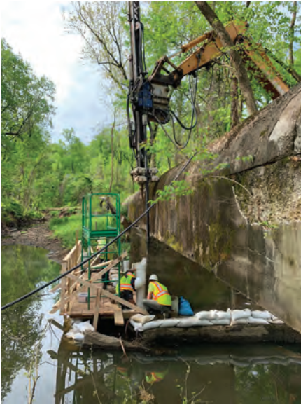
Fig. 4: Micropiles were installed to stabilize the aerial sewer's foundation and tied into the newly placed concrete enlargement of the foundation
