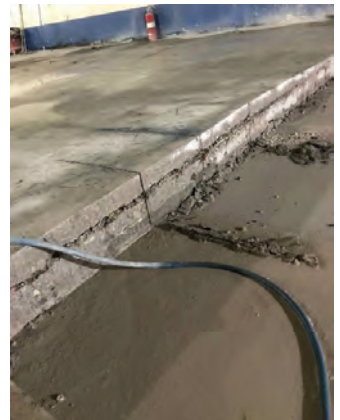
Fig. 3: Separation plane between past repair and original concrete
