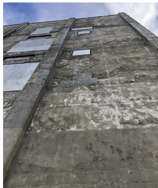
Fig. 3: Elevation showing existing substrate at old patching attempts
