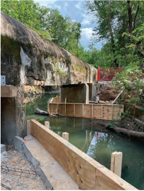
Fig. 2: To provide support for the addition of new piers, a 20-inch-thick foundation was placed on the north and south side of the crossing. Five new concrete piers on piles replaced in-situ piers. New stand-alone piers were installed adjacent to the stream and designed to support the load of the existing piers should they deteriorate
