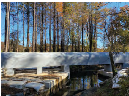
Fig. 7b: The design-build approach allowed the team to collaboratively develop a multifaceted solution for the renewal of the five piers and pipe encasement
