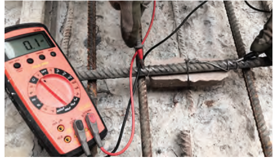
Fig. 11: Galvanic anodes attached to concrete overlay steel in tank floor
