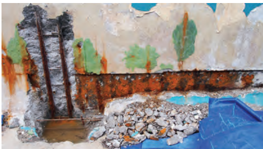
Fig. 4: Example of reinforcing steel corrosion and concrete deterioration
