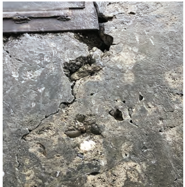
Fig. 7: Area of façade after initial surface preparation showing deep spalls and new construction defects
