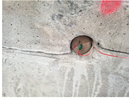
Fig. 10: Type 2A galvanic anode being installed into sound concrete in upper section of tank walls
