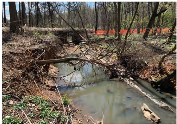
Fig. 1: Severe weather events and significant surge flow precipitated the need for DC Water to implement an emergency design-build repair to address the aerial sewer's structural integrity
