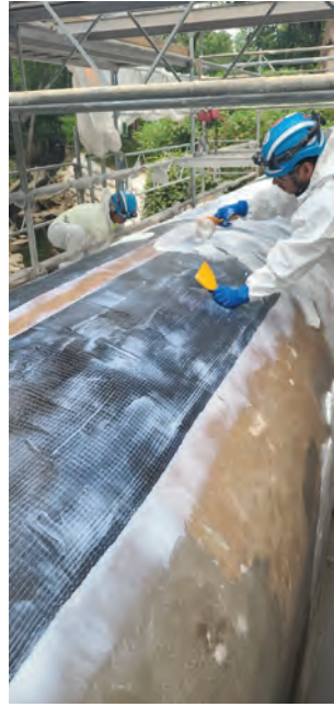
Fig. 3a: State-of-the-art CFRP and GFRP systems were installed to strengthen the unsupported span overtop the creek
