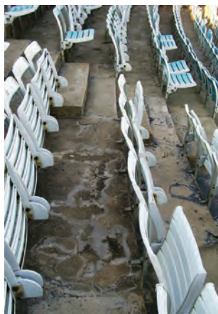
Fig. 1b: Typical deteriorated concrete surfaces at the “Lower Bowl”
