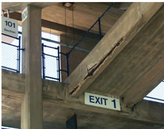
Fig. 1a: Corroded reinforcing steel resulted in spalling of the concrete, posing a significant hazard to patrons below
