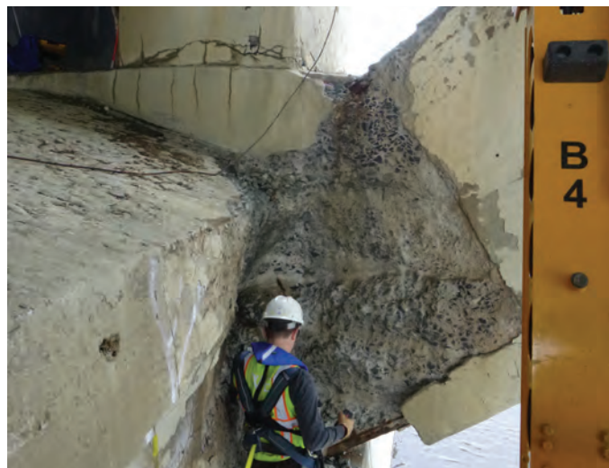
Fig. 4: Deep freeze-thaw deterioration near springline of arch rib below drain discharge (photograph by WJE)
