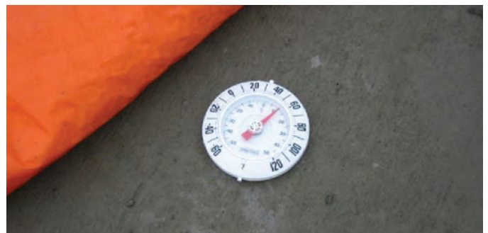
Fig. 4: Insulated blankets help to trap exothermic heat so that hydration and strength gain continues
