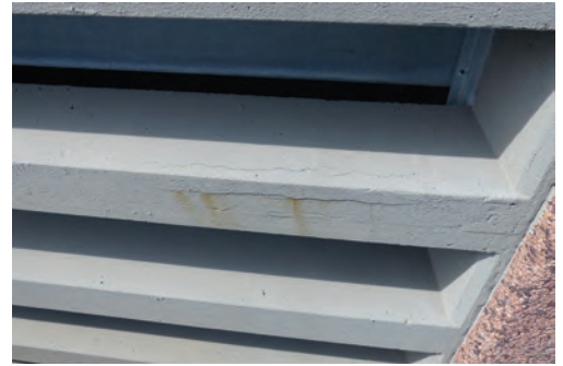
Fig. 5: Concrete deterioration adjacent to prior repairs
