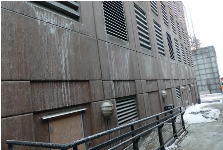
Fig. 6: Salt spray from adjacent elevated roadway
