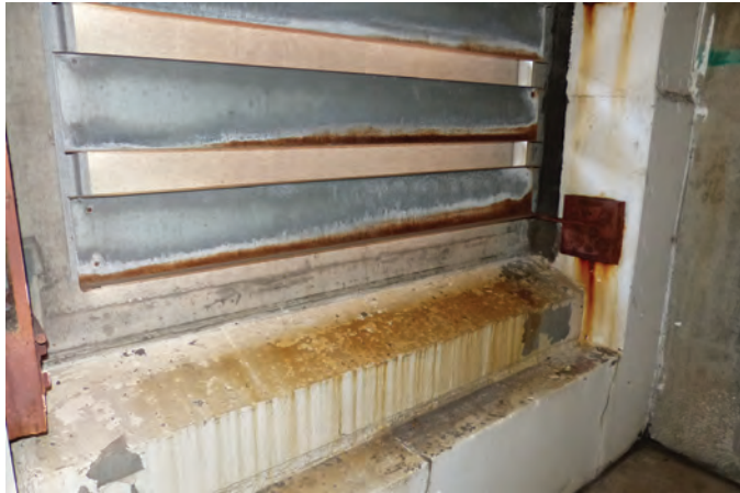
Fig. 11: Channels on interior of garage exhibiting corrosion
