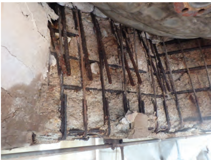
Fig. 4: Spalled concrete with exposed reinforcing on the sides of the octagonal penetration in the upper deck (fractured stirrups are visible)
