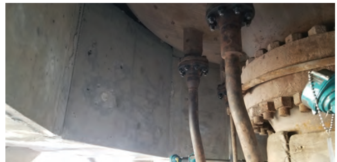
Fig. 11: Completed repair on the sides of the octagonal penetration in the upper deck
