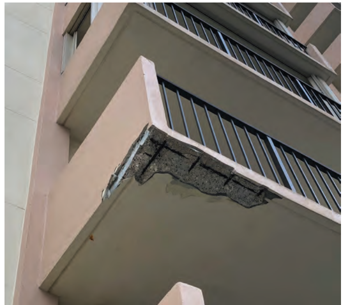
Fig. 3: Typical damage on a structure in Phase 3, Failure—repairs are necessary and corrosion protection will prevent recurrence (Photograph courtesy of No Corrosion, LLC, West Palm Beach, Florida)
