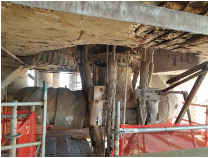
Fig. 2: View of octagonal penetration in upper deck and piping associated with the catalytic reformer
