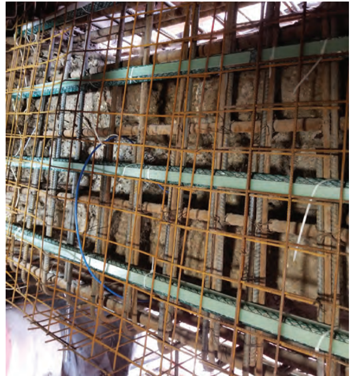
Fig. 10: Welded wire reinforcing, galvanic anodes, and concrete maturity meter in repair area
