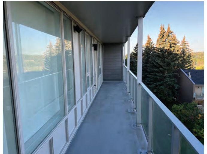
Fig. 2: Typical TDC installed on balcony
