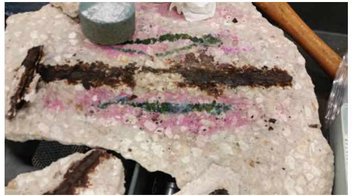
Fig. 6: Carbonation testing of concrete samples using phenolphthalein indicated extensive carbonation
