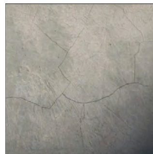
Fig. 3: Typical cracks in concrete
