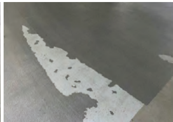
Fig. 10: Intercoat adhesion failure between topcoat and base coat
