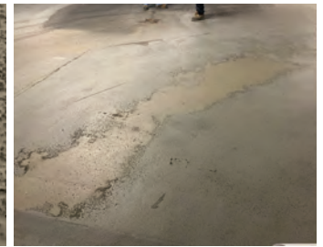
Fig. 13: Excessive wear through entire coating system
