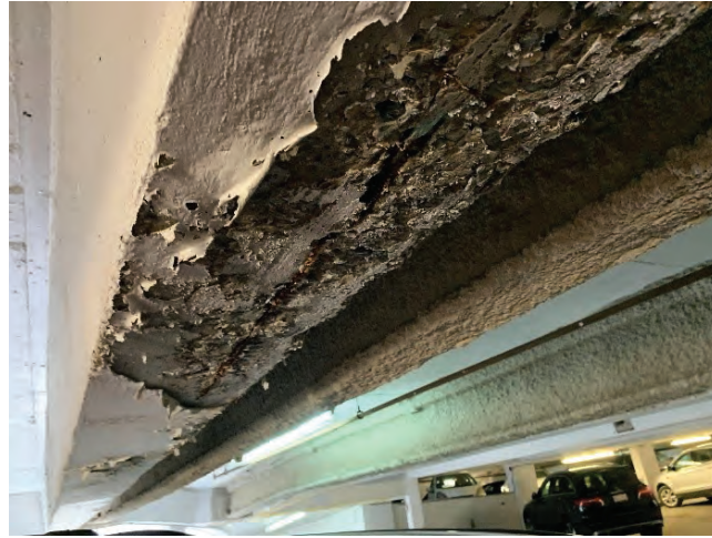
Fig. 5: Concrete deterioration on bottom surface of beam
