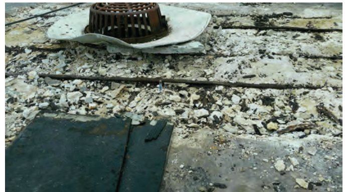
Fig. 4: Photograph of the roof. Note the complete failure of the roof membrane and extensive corrosion of the exposed reinforcing steel
