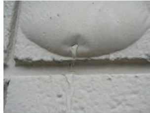
Fig. 4: Water dripping from behind blistered coating
