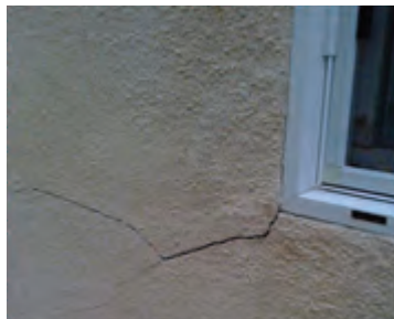
Fig. 1: Crack in exterior stucco
