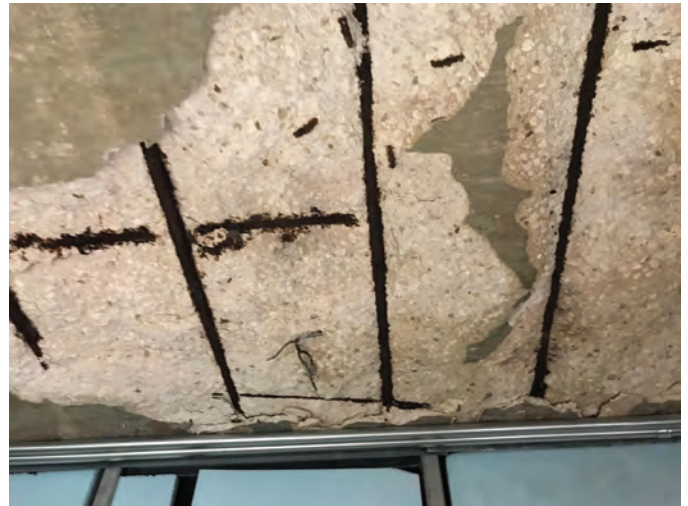
Fig. 3: Typical condition of the undersides of the 4th floor and roof
