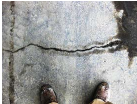
Typical negative moment crack over beams
