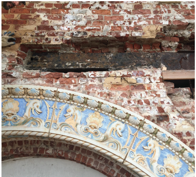
Fig. 3: Steel deterioration near window openings
