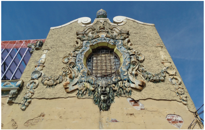
Fig. 2: Water damage of ornamental terra cotta pieces
