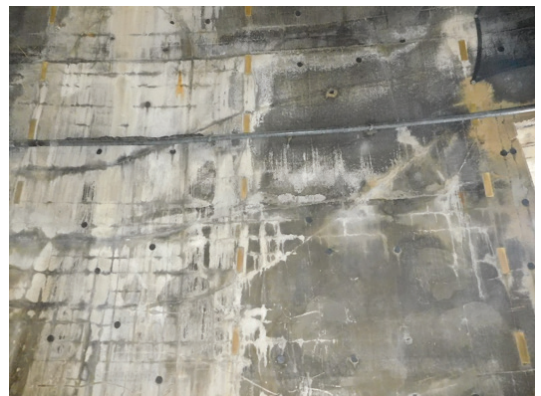
Fig. 4: Shadowing of shotcrete created voids behind welded wire fabric reinforcement and post-tensioned tendons
