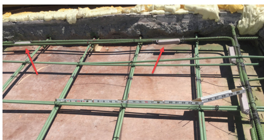
Fig. 9: Type 1A embedded galvanic anodes were installed in traditional concrete repairs and skylight closure pours
