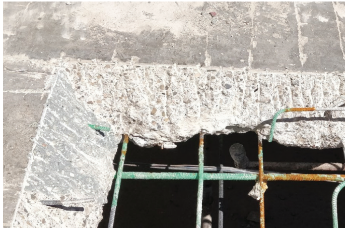
Fig. 1: Existing reinforcing steel corroded at the edge of a previous repair (incipient anode effect)
