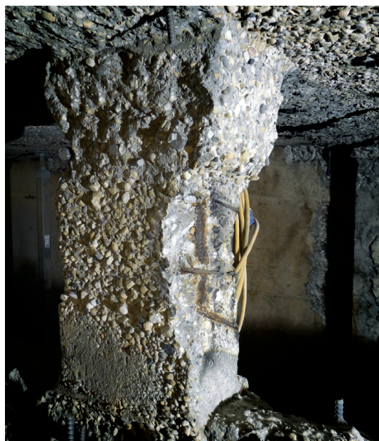
Fig. 2: Column and ceiling deterioration
