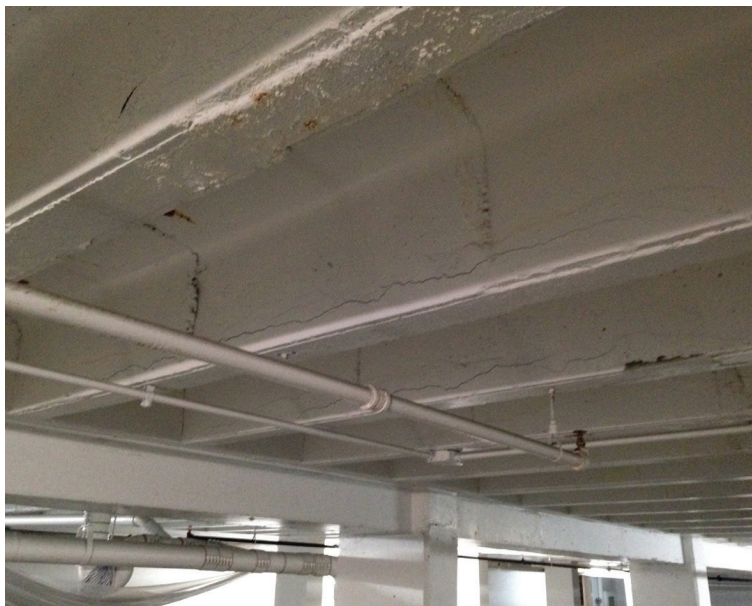
Fig. 1: Concrete deterioration at existing concrete joist.
