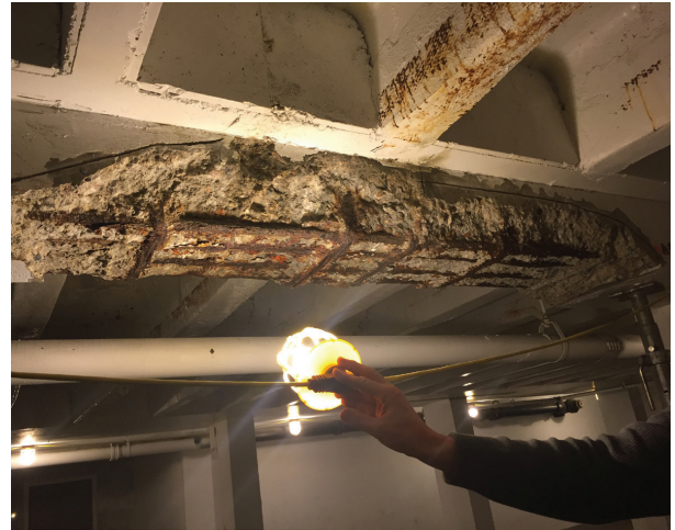
Fig. 2: Concrete deterioration at existing concrete beam.
