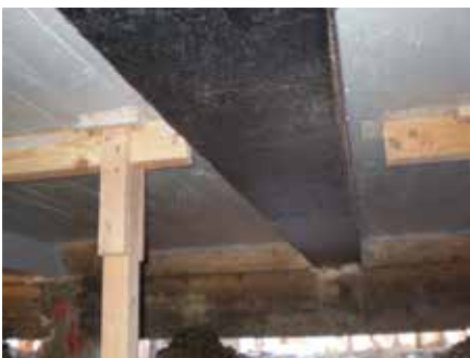
Fig. 9: Girder after application of CFRP and slab after application of epoxy coating (note areas of shoring that required later touchup)
