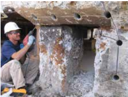
Fig. 7: Anodes installed throughout to combat the high chloride content in the concrete
