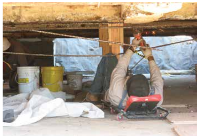
Fig. 4: A worker works off his back on a mechanics crawler to grind and clean the reinforcing steel
