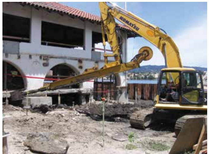
Fig. 3: Modified excavation equipment to remove the mucky soil under the supported slab
