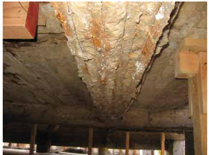
Fig. 2: Extensive spalling of the beams, girders, and slabs caused by severe corrosion of the reinforcing steel
