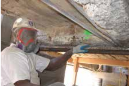
Fig. 6: Significant demolition required to remove spalled concrete and expose corroded reinforcing steel
