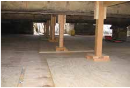
Fig. 5: Work platform and shoring installed ahead of demolition (note corroded steel throughout and the tight working conditions)
