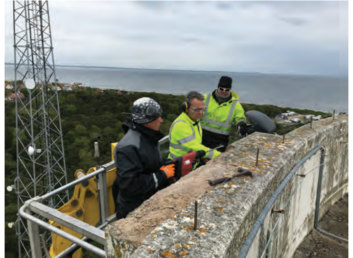
Fig. 2: Examining damaged concrete and corroded reinforcement at the top of the reservoir
