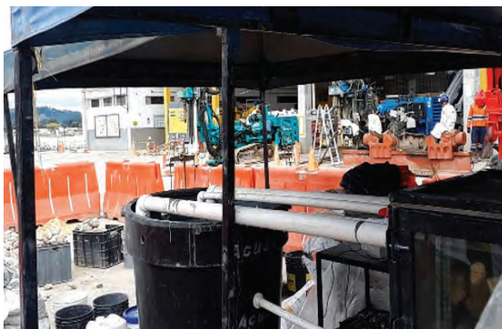
Fig. 11: Overflow from the large-scale mockup was captured and weighed to determine the amount of washout
