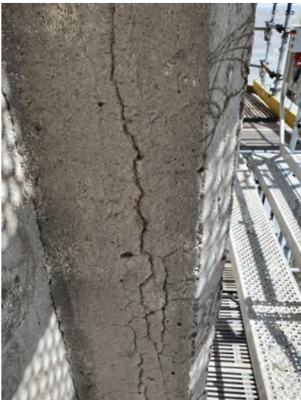
Fig. 5: Close-up of visible cracks after sandblasting the existing paint off
