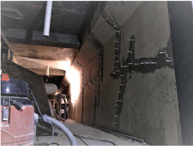
Fig. 3: Epoxy injection of wall cracks (photo courtesy of Simpson Gumpertz & Heger, Inc.)
