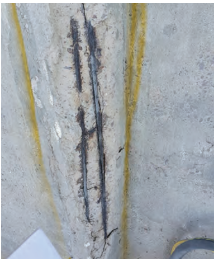
Fig. 6: Splintering concrete and exposed rebar in damaged area
