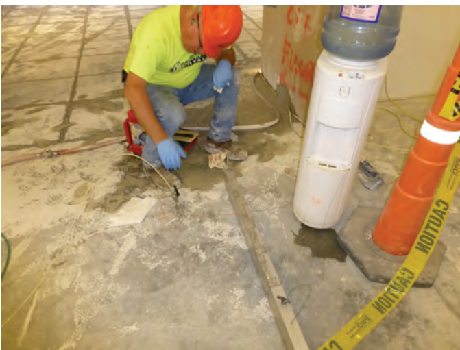
Fig. 4: Epoxy injection of a floor slab crack (photo courtesy of Simpson Gumpertz & Heger, Inc.)
