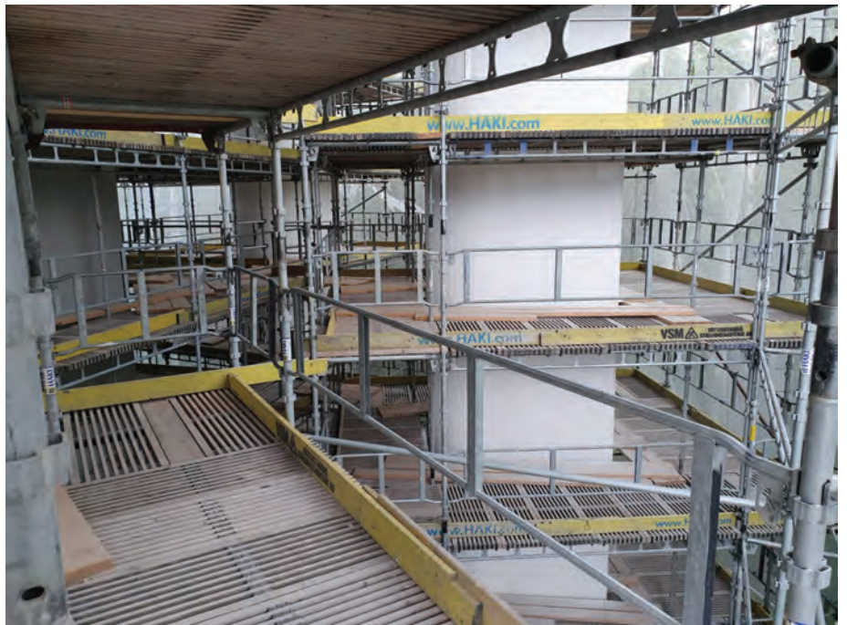
Fig. 9: After washing all surfaces, protective paint was sprayed onto the entire structure
