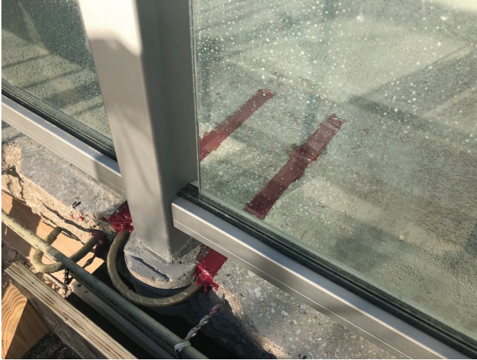
Fig. 12: Strengthening of a deficient railing anchorage
