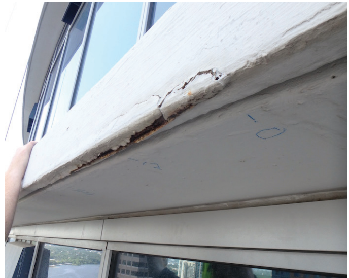
Fig. 4: Corrosion-induced damage at an exposed slab edge
