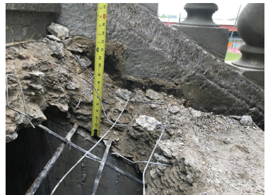
Fig. 4: Condition of the existing structural slab with topping slab removed, illustrating the lack of waterproofing between the slabs
