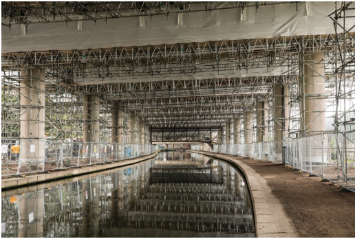
Fig. 6: Concrete repairs and installation of cathodic protection on the underside of the viaduct
