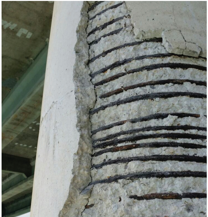
Fig. 2: Column deterioration during the bridge inspection
