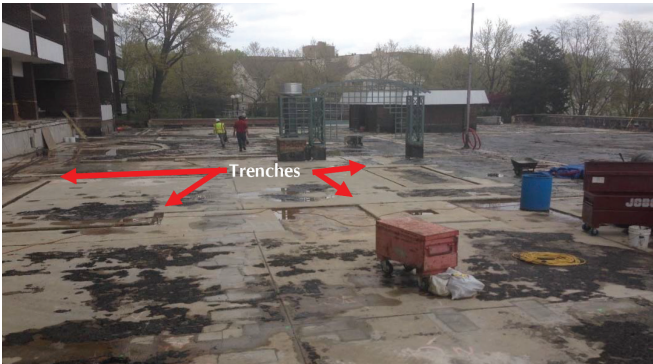
Fig. 5: Plaza demolition revealed topping slabs that overlaid the structural deck
