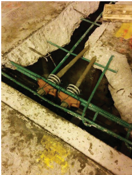
Fig. 8: New encapsulated PT anchors at expansion joint
