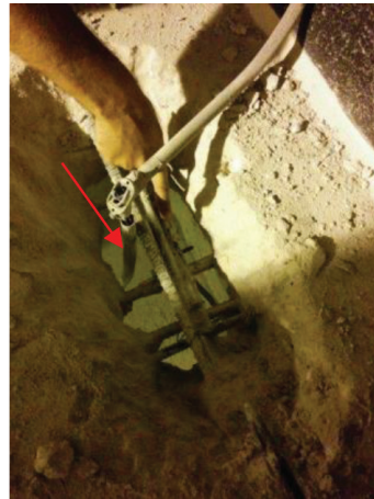
Fig. 3: Electrical conduit (red arrow) and PT cables from top of slab
