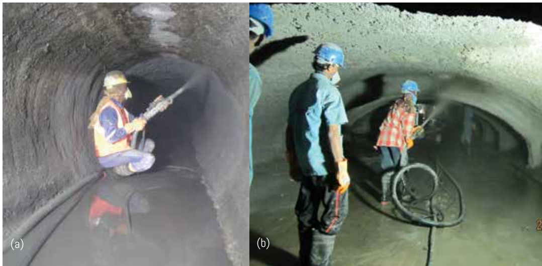
Fig. 12: Spraying two-component mineral based mortar system to form a lining (a and b)
