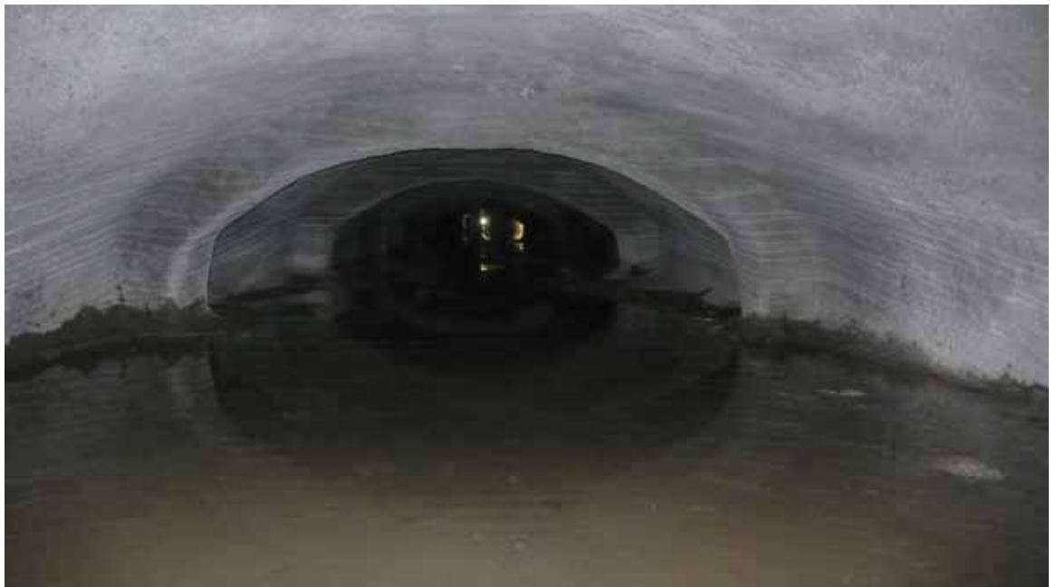
Fig. 1: Completed repair of the storm water drains in the City of Mumbai, India, that are more than a century old and were constructed of brick arch masonry during the British Era
