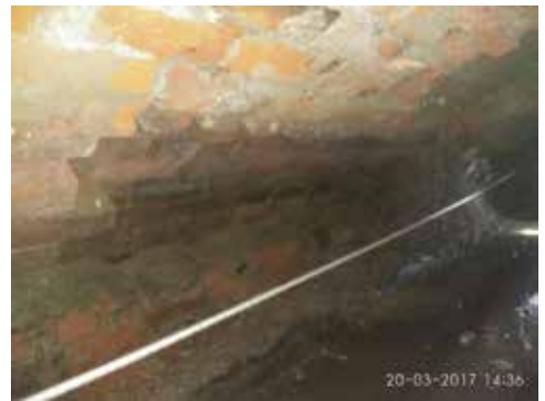
Fig. 2: Delamination and spalling of brick lining
