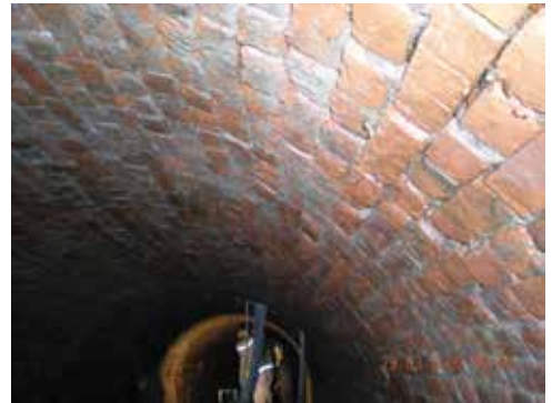
Fig. 3: Erosion of mortar joints
