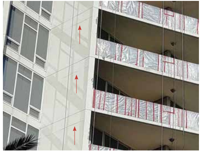
Fig. 2: Cracks in stucco on every floor at bottom of turndown beam to top of wall
