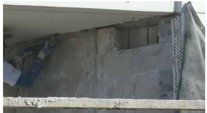
Fig. 4: CMU reinforced cells missing grout
