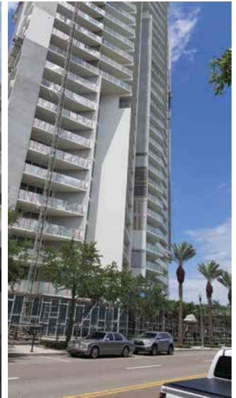
Fig. 8: Stucco replacement, CMU grouting, guardrail protection, overhead protection, and mast climber/swing stage access
