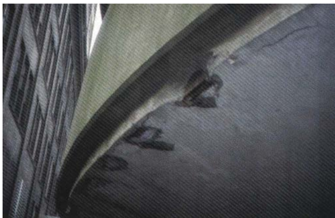
Fig. 2: Original slab edge deterioration
