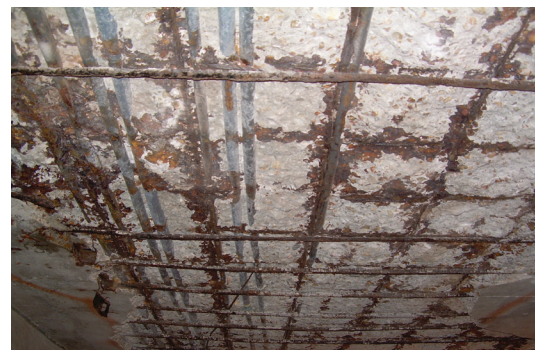
Fig. 3: Underside spalling and steel corrosion
