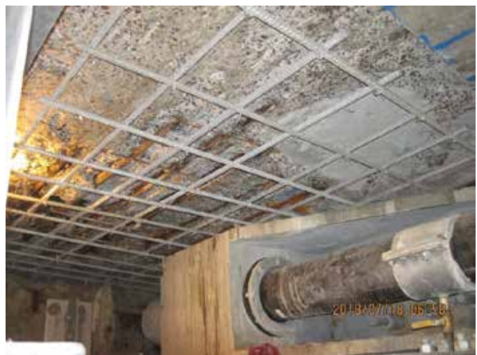
Fig. 7: Underside heavy duty slab repair prior to adding forms, concrete and steel deck and transverse beams
