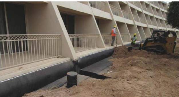
Fig. 7: Foam blocks and backfilling in progress after completion of waterproofing repairs along the expansion joint
