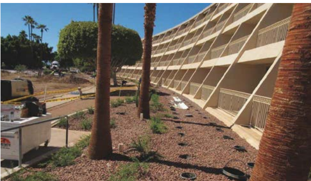
Fig. 8: Completion of repairs with new landscaping in front of the hotel building
