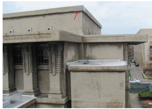
Fig. 2: Concrete cracking and deterioration on exterior walls and cantilevered roof slabs—loose spall at corner of parapet wall (arrow) was removed and covered to address potential falling hazard prior to restoration
