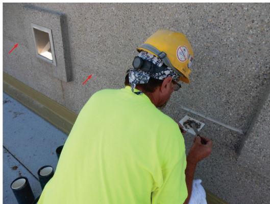
Fig. 7: Routed and sealed construction joint repair (arrows point to completed joint repair)—crack repair was similar
