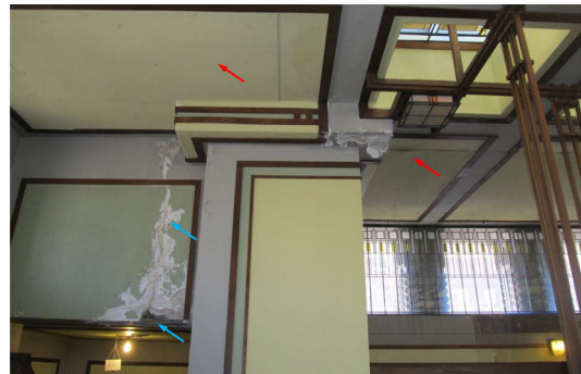
Fig. 3: Concrete deterioration of concrete beam (blue arrows) and water damage to plaster finish at interior of Unity Temple Sanctuary—roof slab underside delaminations were removed and covered with plywood (red arrows) to address potential falling hazards prior to restoration
