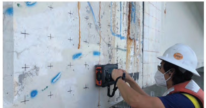
Fig. 3: Horizontal GPR scanning on a 3 in (75 mm) grid (vertical scans were also completed) for 3D GPR image
