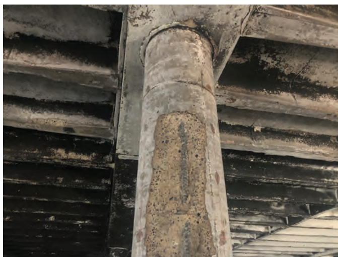
Fig. 3: Spalling that occurred on a concrete column due to fire exposure
