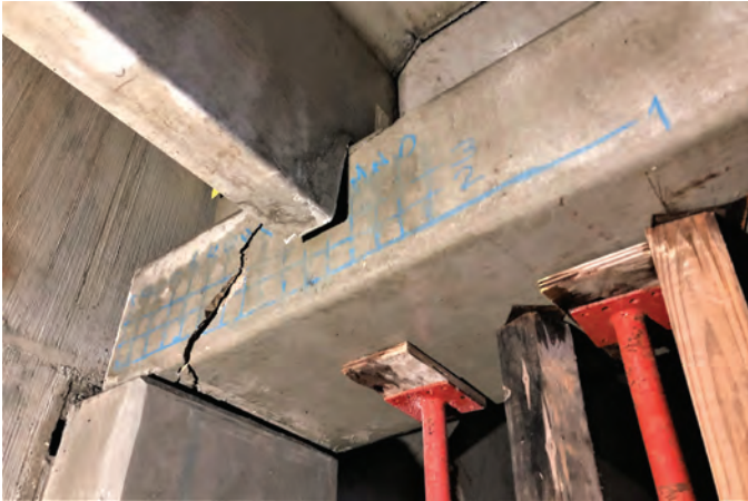
Fig. 6: Girder cracking/faulting near support
