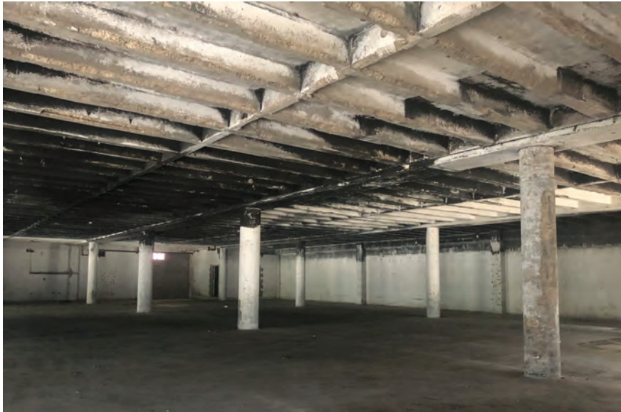
Fig. 1: A reinforced cast-in-place concrete structure that was damaged due to a fire event
