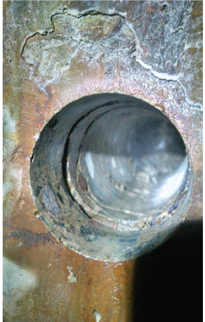
Fig. 6: Core hole showing delaminations in the concrete
