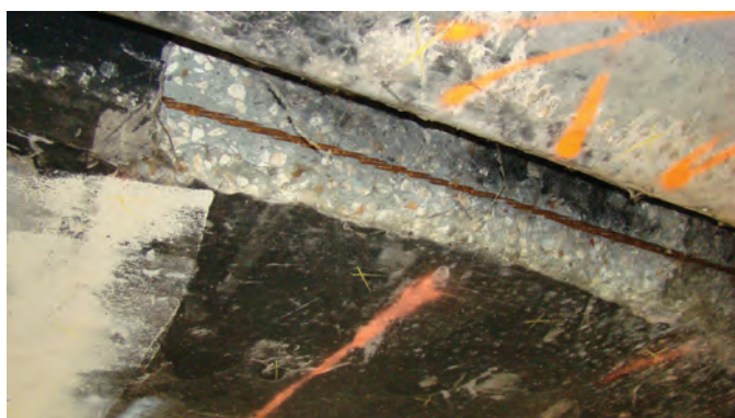
Fig. 4: Spalling of concrete box beam and exposed prestressed strand due to fire event
