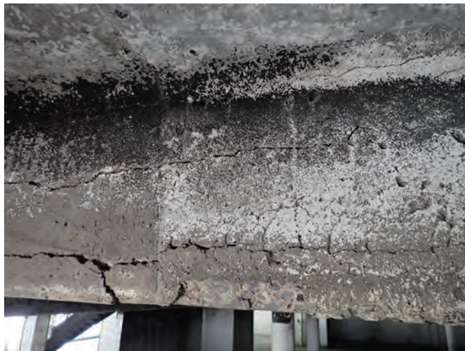
Fig. 2: Cracking along the length of a reinforced concrete joist due to fire exposure
