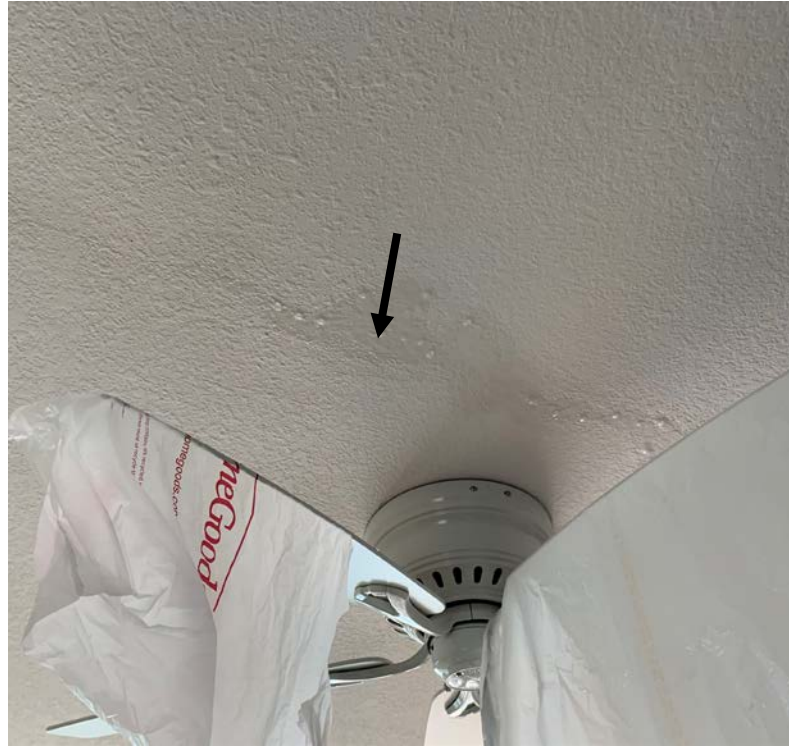
Leak in Middle of Living Room in Ceiling
