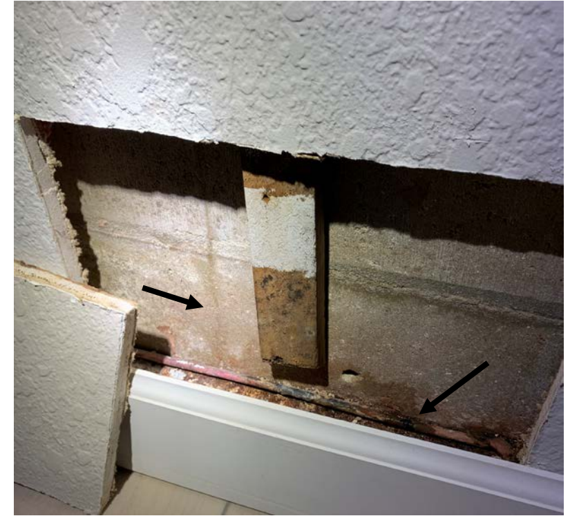
Water at Inside Face of Exterior CMU Wall
