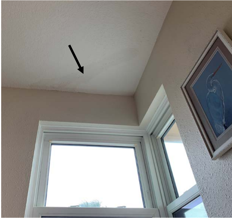
Leak at Southeast Corner in Ceiling
