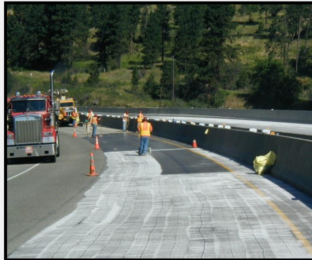
Remove excess epoxy and immediately apply fine sand into the wet epoxy
