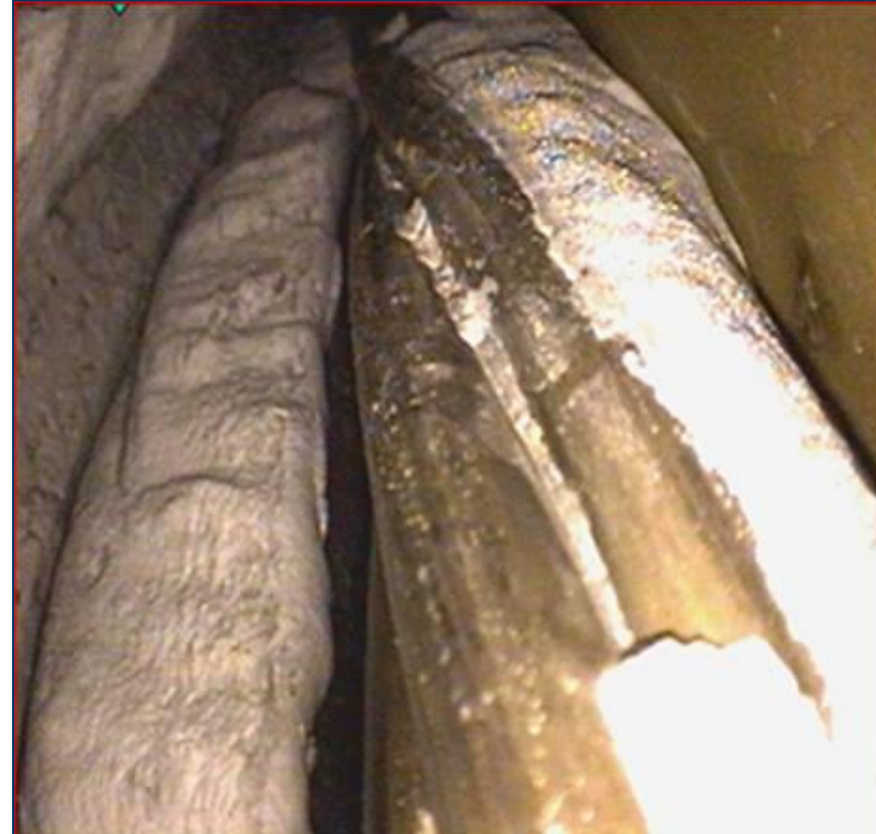
Poorly Grouted Duct – Tendons Exposed (from Video borescope)
