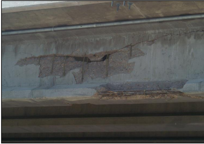
Bridge Girder with Cracks and Spalls
