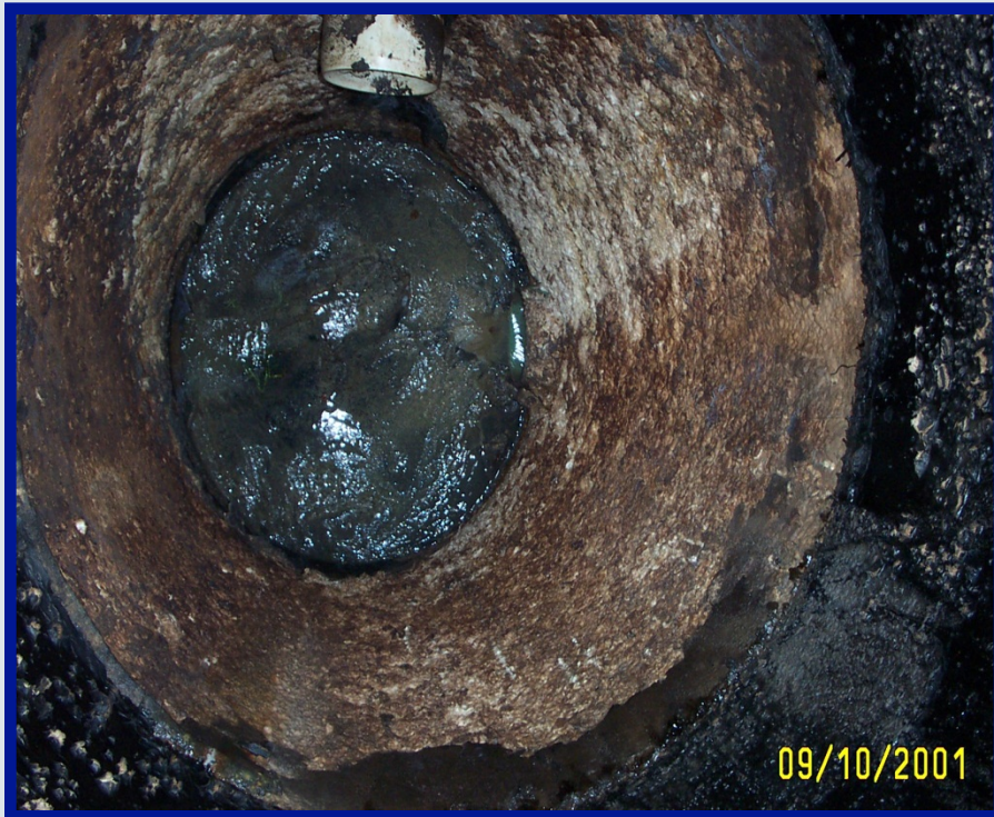
Precast Manhole with Failure of Existing Coating
