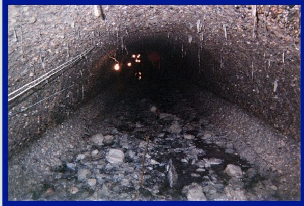
Ongoing Disruptive Phenomena is apparent with existing portland cement based materials
