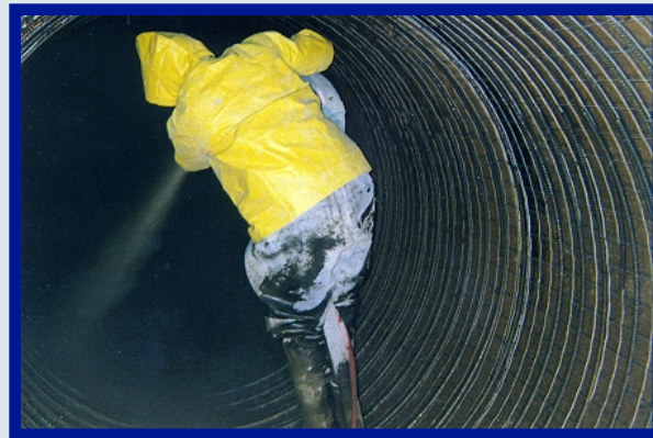
The clean, prepared, and reinforced structure receives a 100% Calcium Aluminate mortar installation
