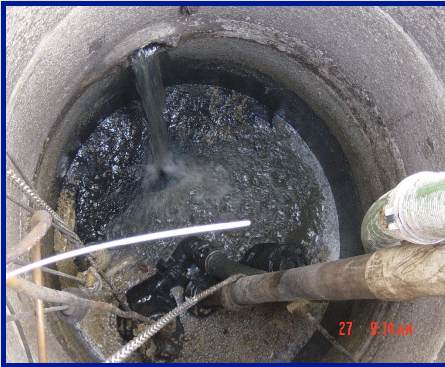
Existing Wet Well
