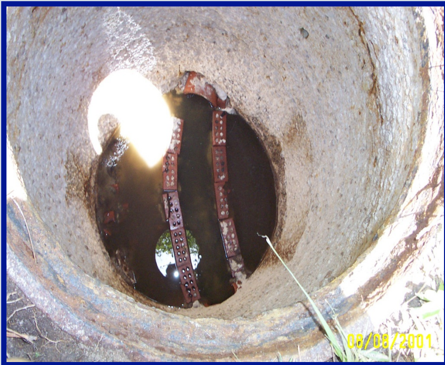
Deteriorated Precast Manhole with Bench & Invert Problems
