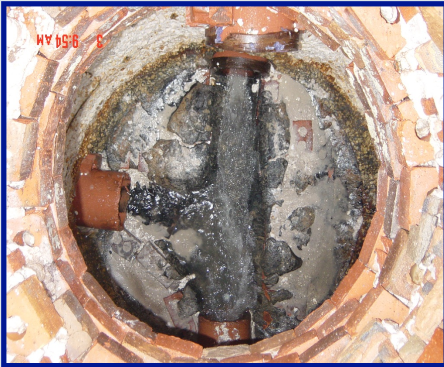
Existing Brick Manhole with Tidal Infiltration
