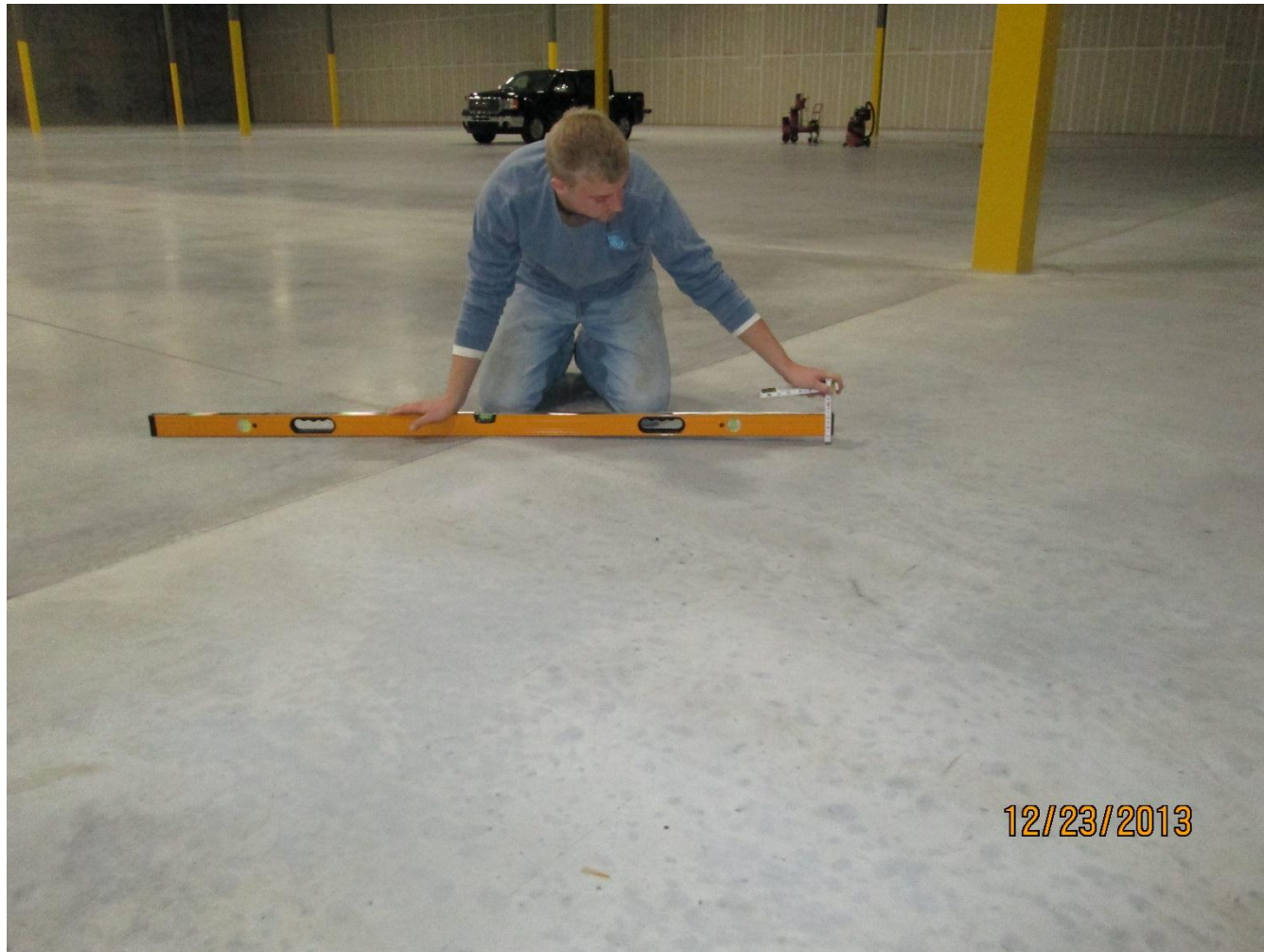
Curling Noted Across Joints
