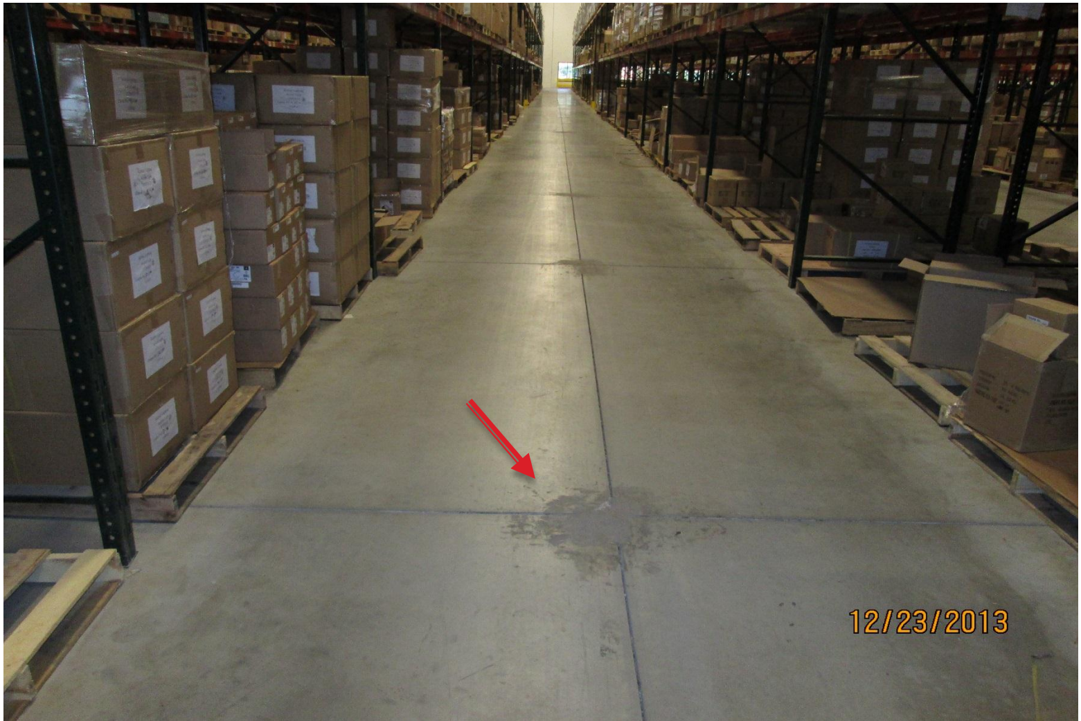
Distressed Warehouse Floor Slab
