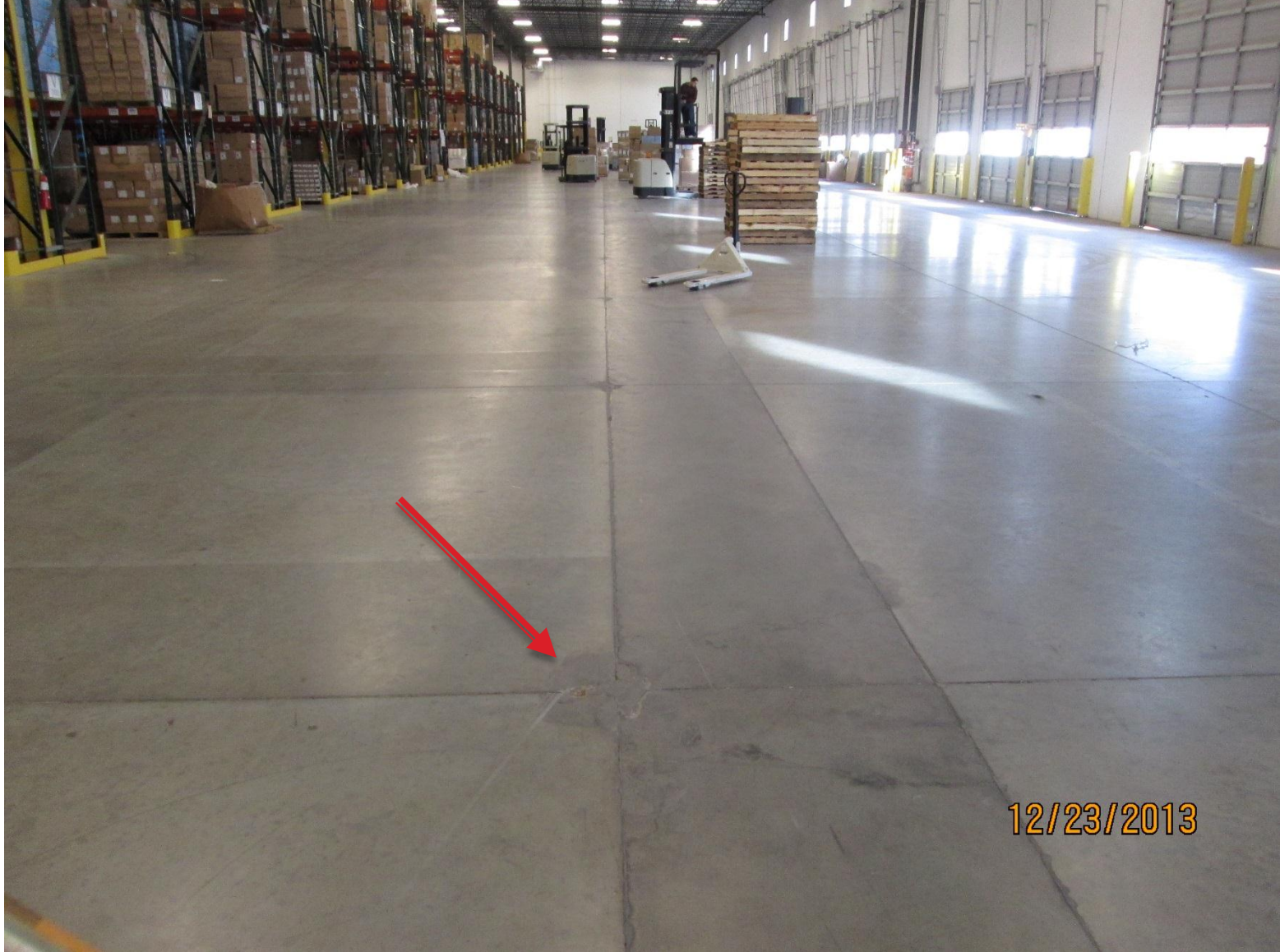
Distressed Warehouse Floor Slab
