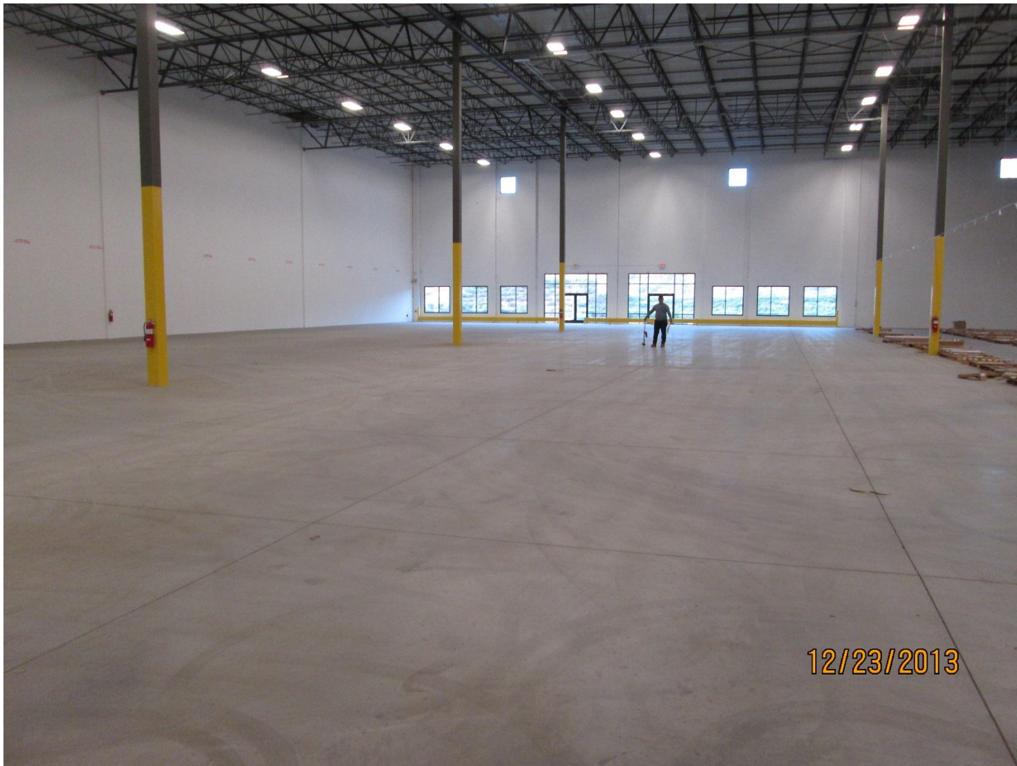
Curling Noted Across Joints
