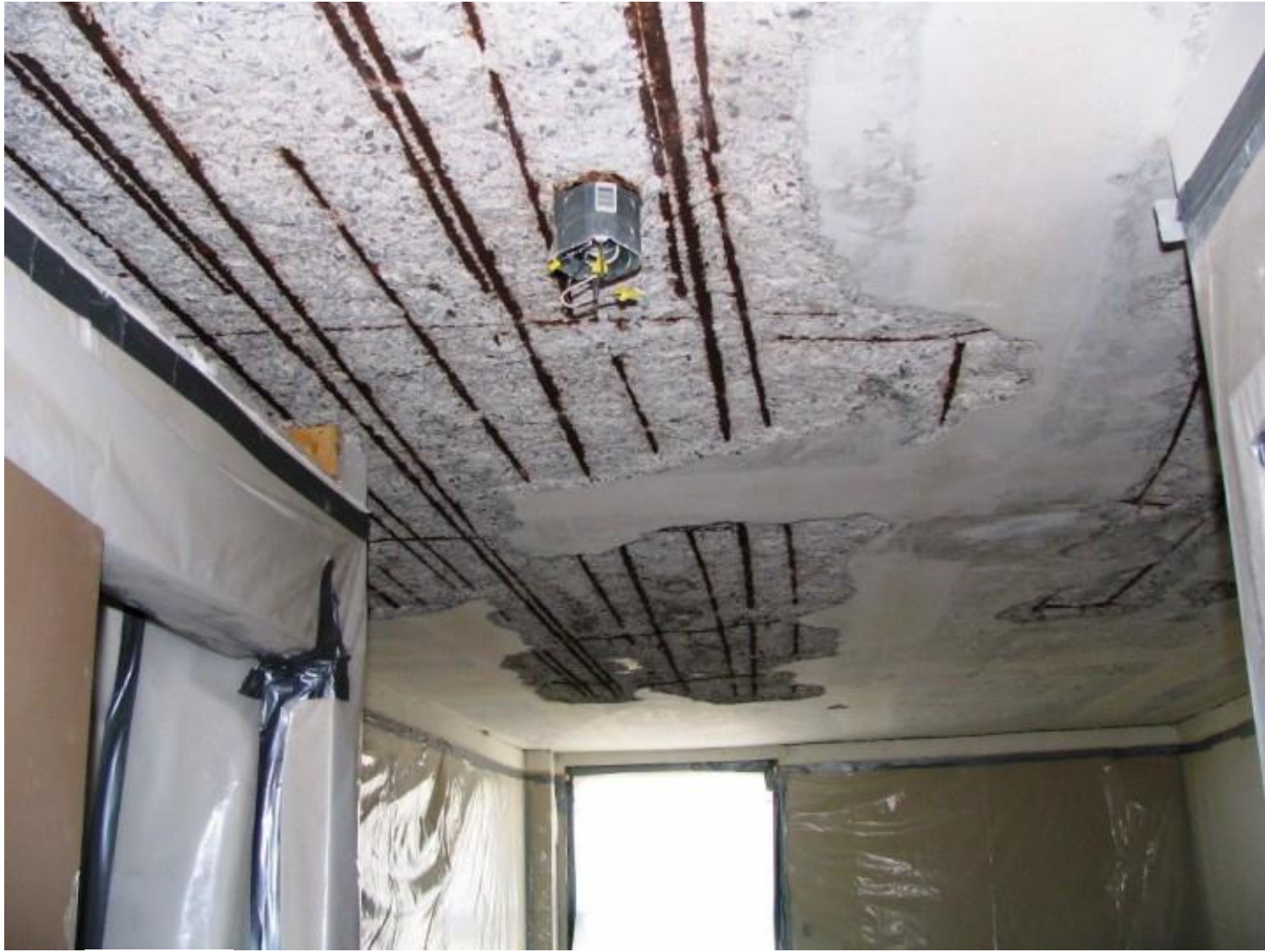
Overall of severe spalling of underside of roof slab *POSTER*.
