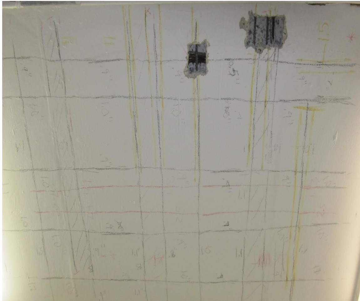
3D scan transferred to slab and chipped out excavations to measure bar size
