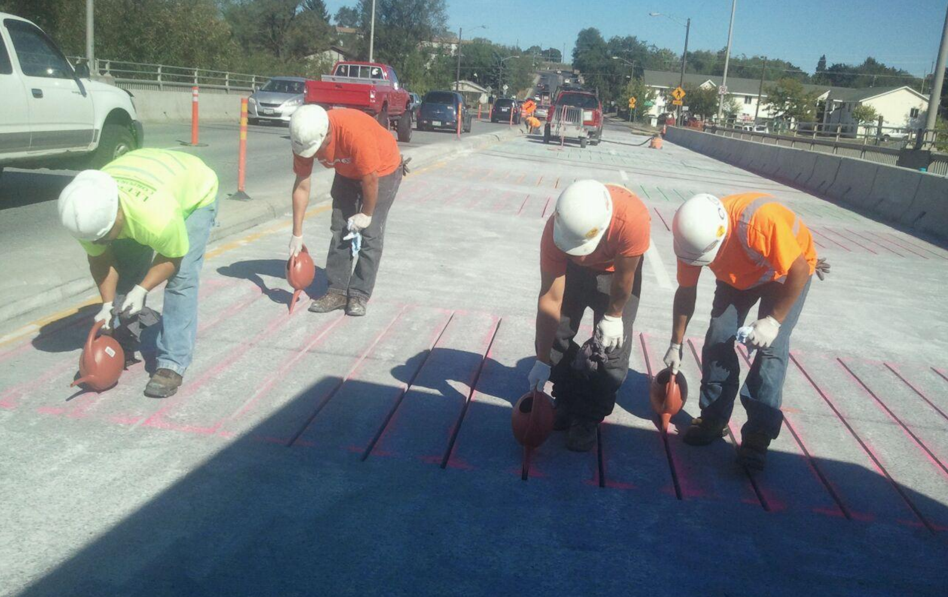
FILLING THE SLOTS WITH EPOXY TO THE TOP OF THE STRUCTURAL SLAB
