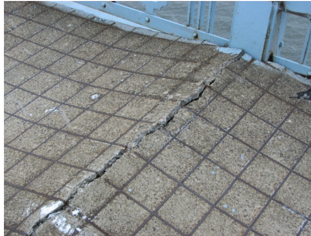
SECTION OF DOWNSTREAM SIDEWALK HAS CRACK & IS HEAVED CAUSING A 1 FT RISE & CREATING TRIPPING HAZARD @ VERTICAL MEMBER 19
