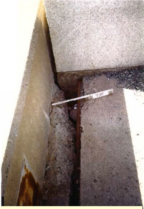
NORTH END OF SPAN 11 AT PIER 11 NOTE: 2' X 6" WIDE SPALL IN WEST SIDEWALK
