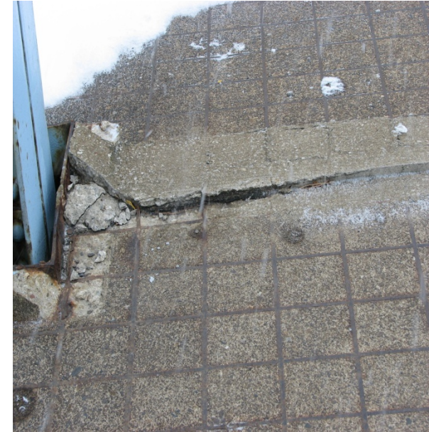
MINOR TRIPPING HAZARD OF DOWNSTREAM SIDEWALK @ VERTICAL MEMBER 6
