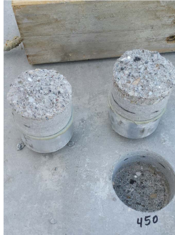
Failure at substrate
