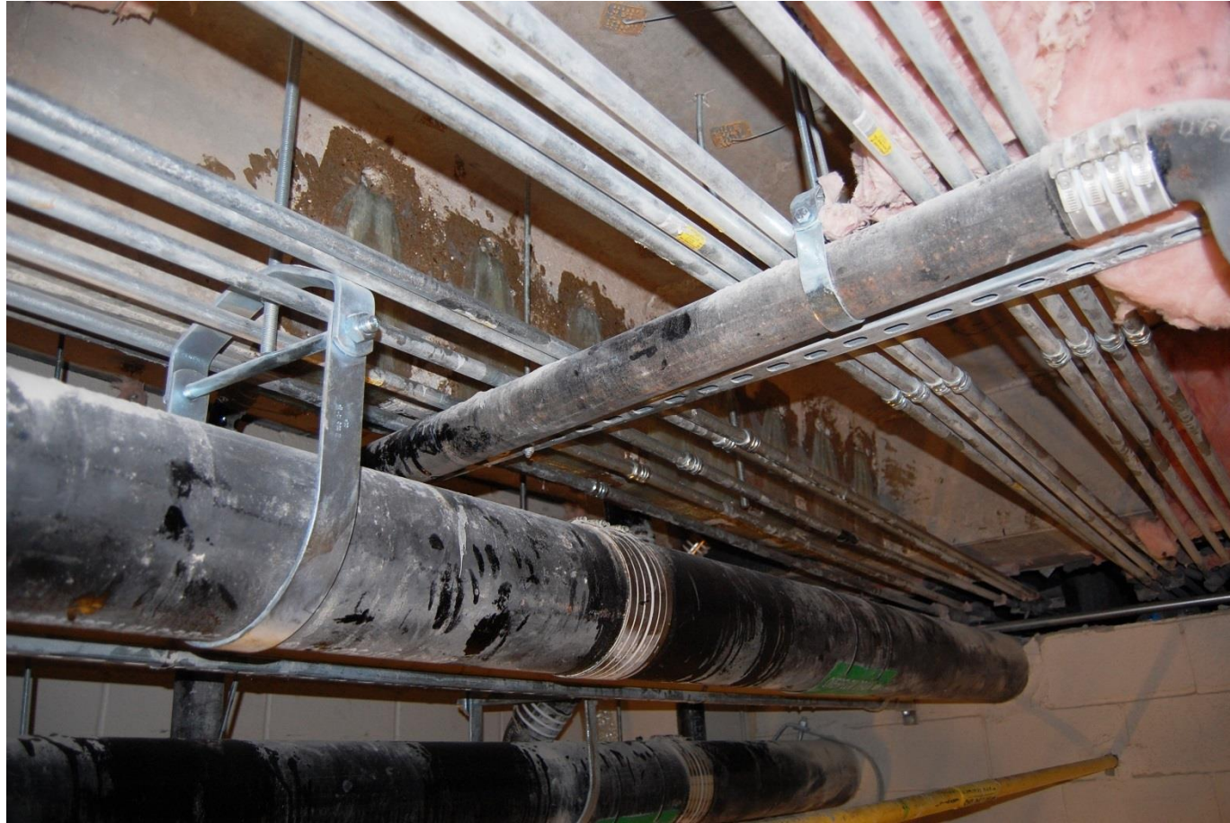
Difficulty of Access
