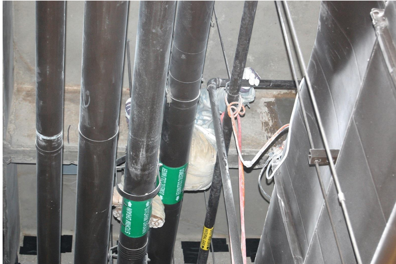
Difficulty of Access
