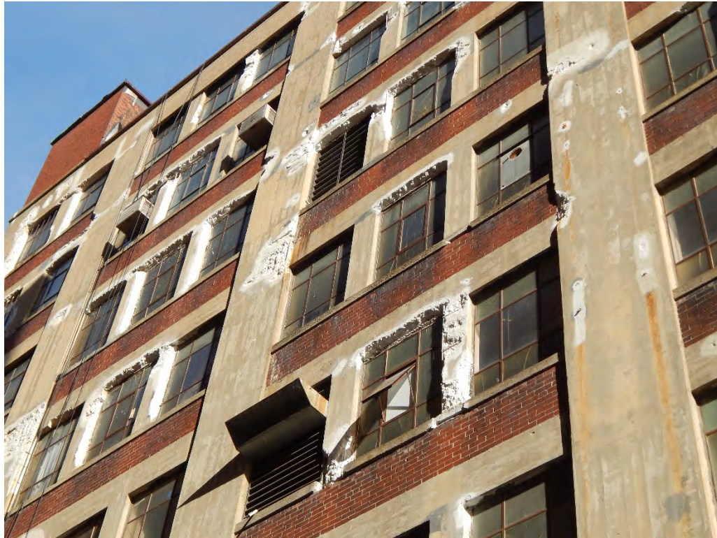
At Left: Partial view of the South (rear) Elevations and associated spall areas.
