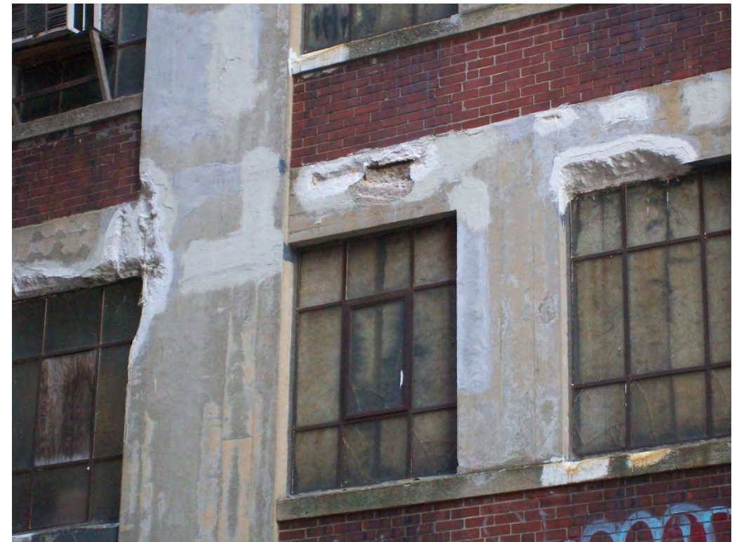
At Right: Close-up view, typical spalling conditions throughout the building.
