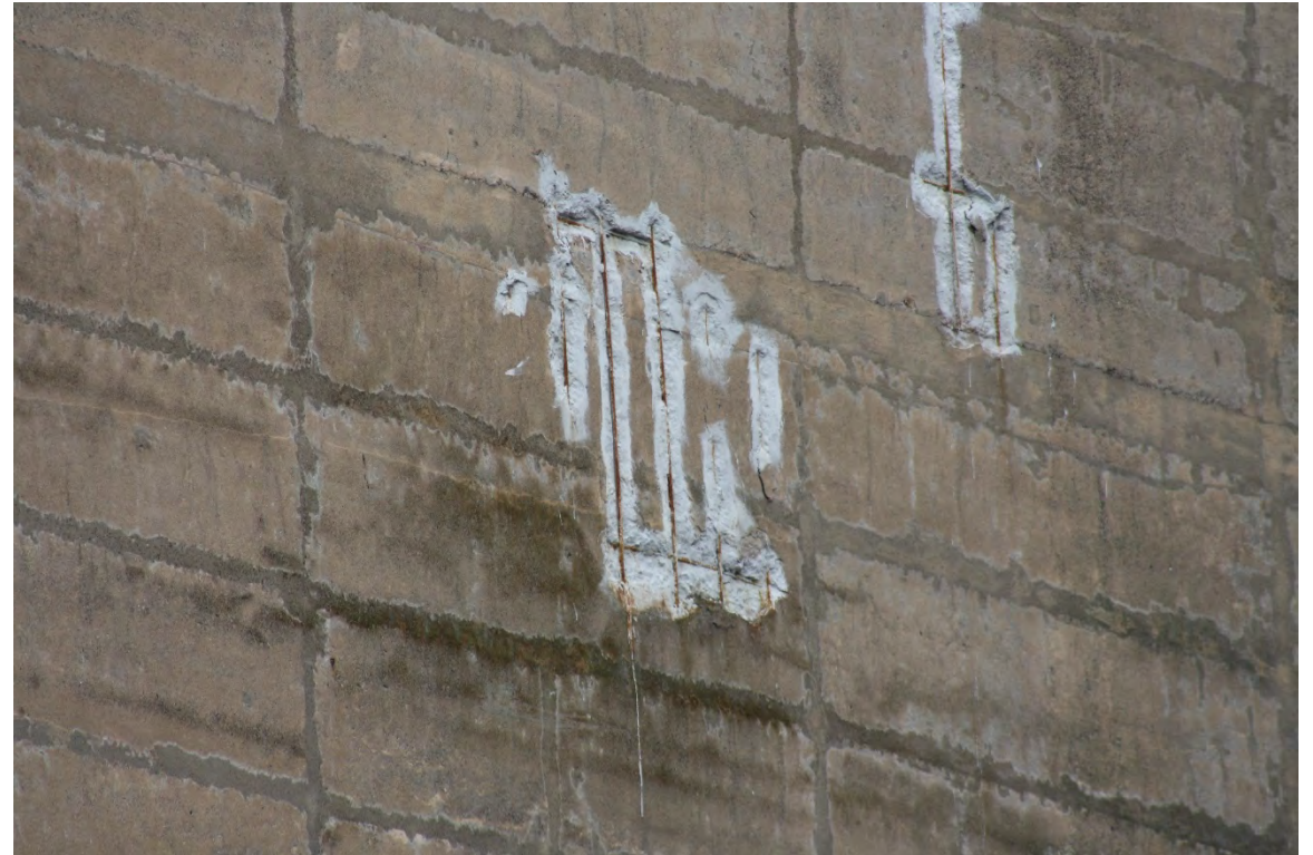
At Right: Representative spall locations.
