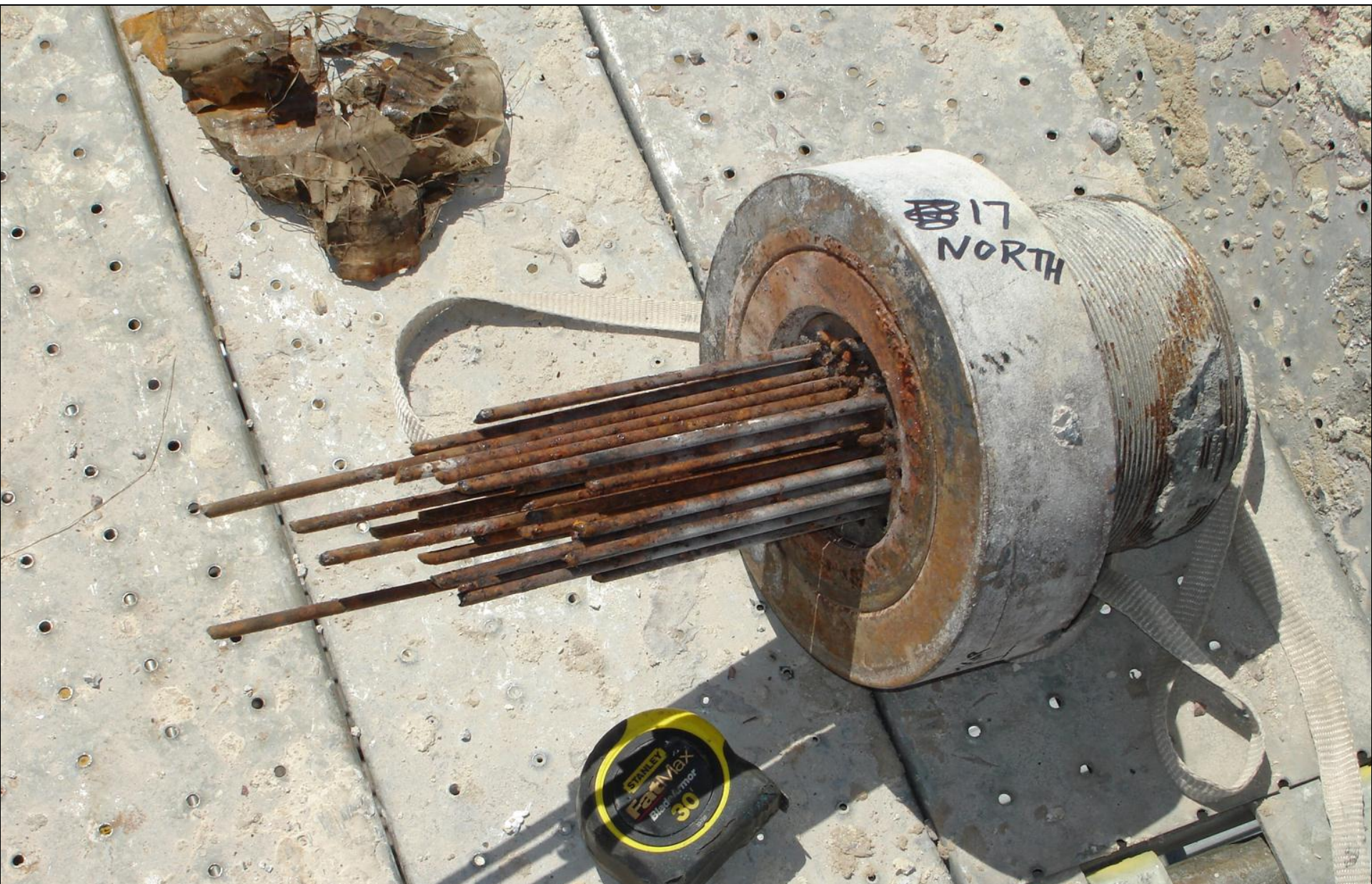
Failed end anchorage of post-tensioned cable. Failure caused by Hydrogen Embrittlement. Post-tensioned force 420,000 pounds.
