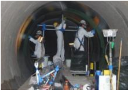
Pipe, Costa Rica
