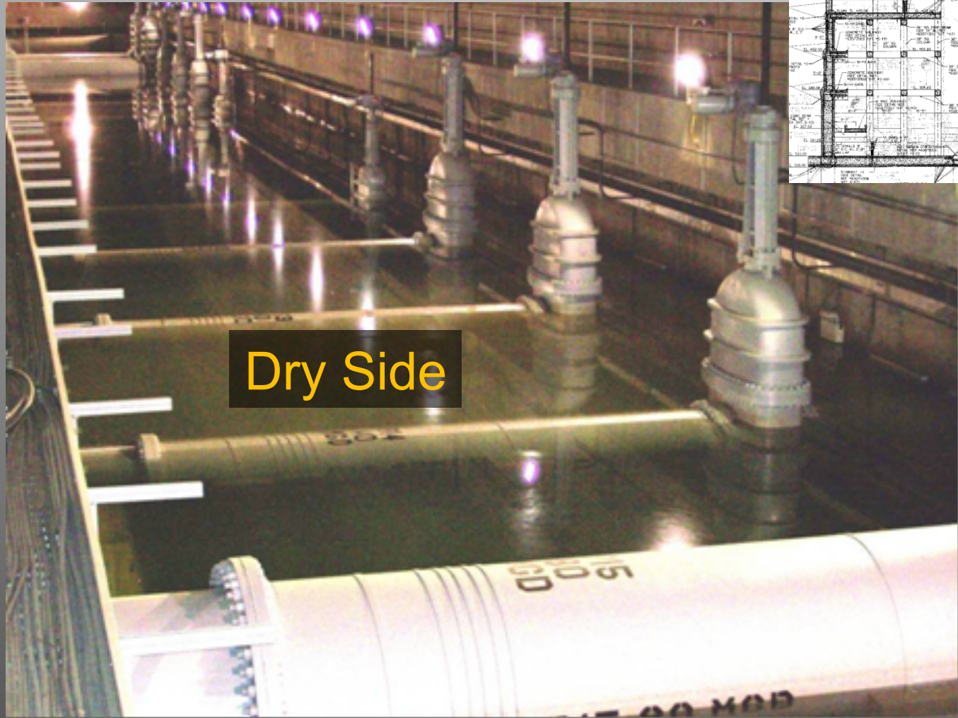
Groundwater flooded the dry side of the vault.
