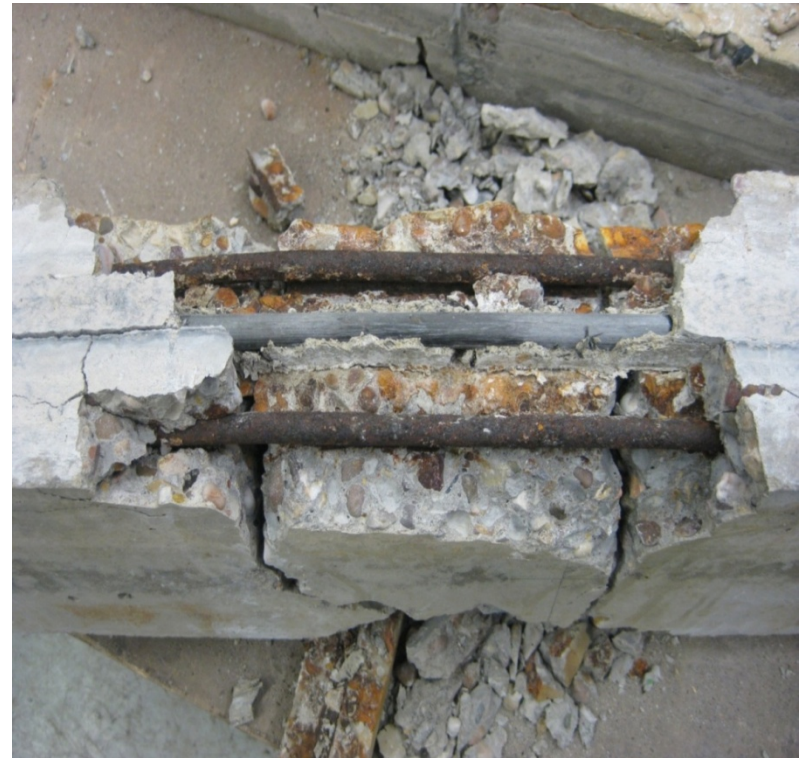
CFRP rod - after testing Failure at rod:concrete interface
