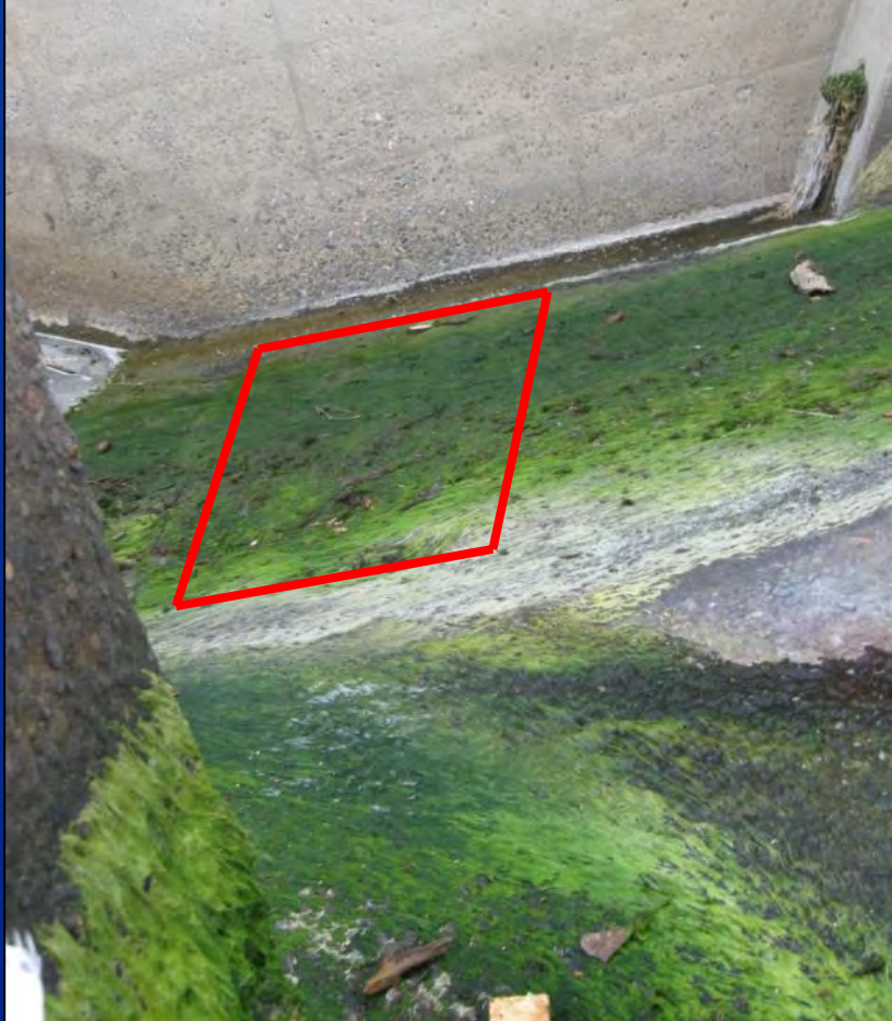
Grade X - Missing
